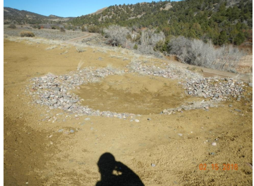
Photo 4: View of silt trap in the eastern portion of the project area that is filling with sediment and needs maintenance.
