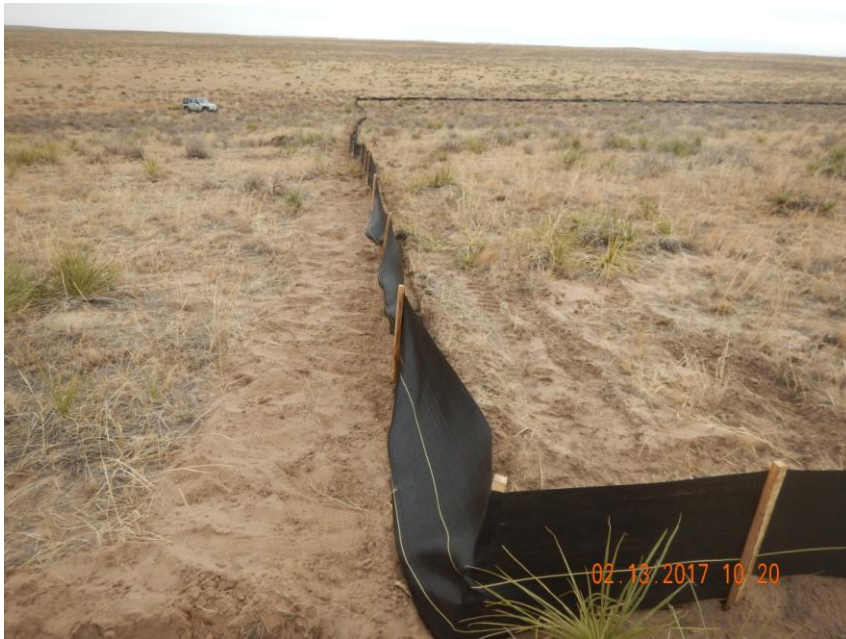
Figure 1: Photo taken from the southwest corner of the location, facing north. Photo shows silt fence used as a stormwater and sediment control BMP has been installed prior to construction/surface disturbing activities.
