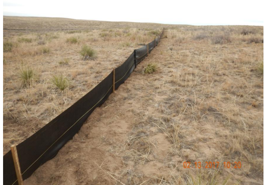
Figure 2: Photo taken from the southwest corner of the location, facing north. Photo shows silt fence used as a stormwater and sediment control BMP has been installed prior to construction/surface disturbing activities.
