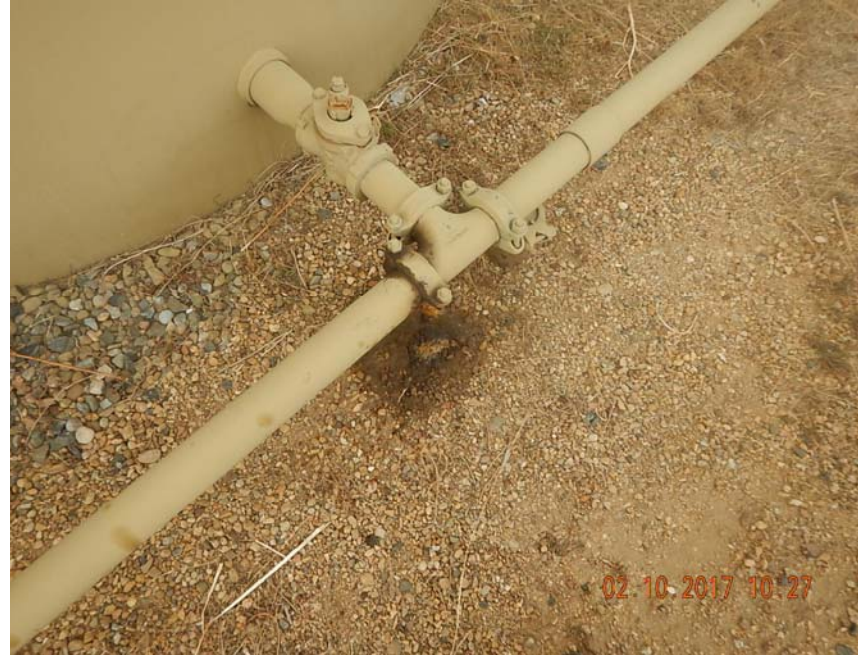
Photo 4: Stained soil at loadout, W tank
