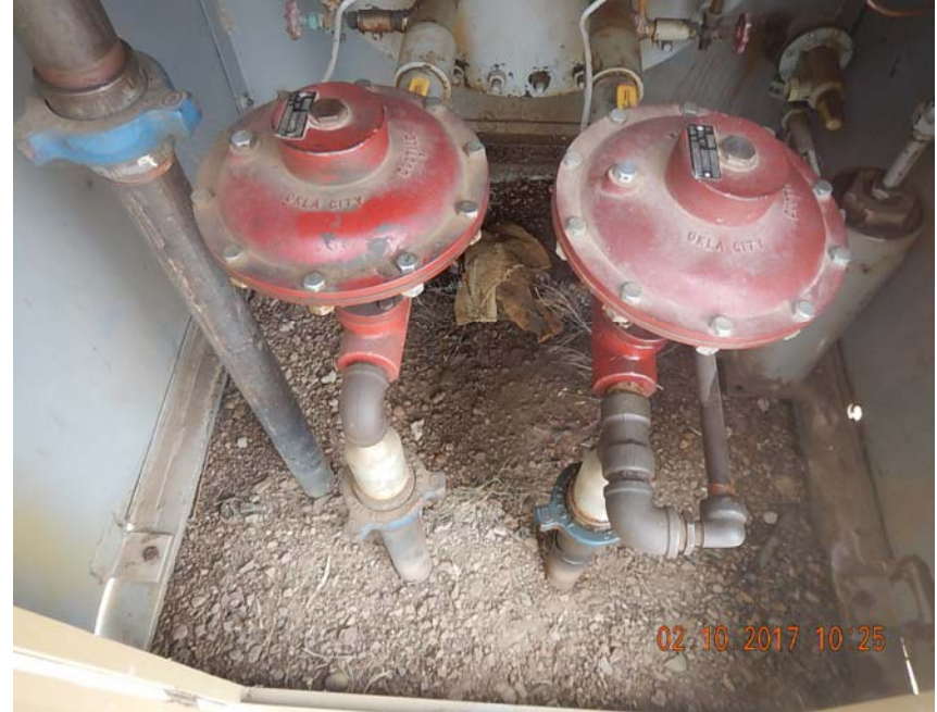
Photo 7: Stained soil in separator house
