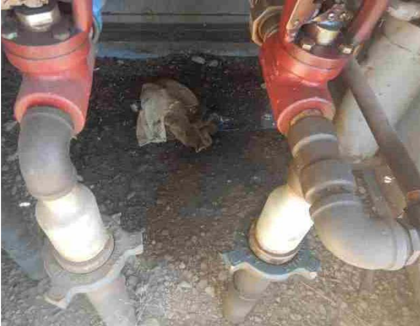
Prior inspection photo for comparison purposes only
