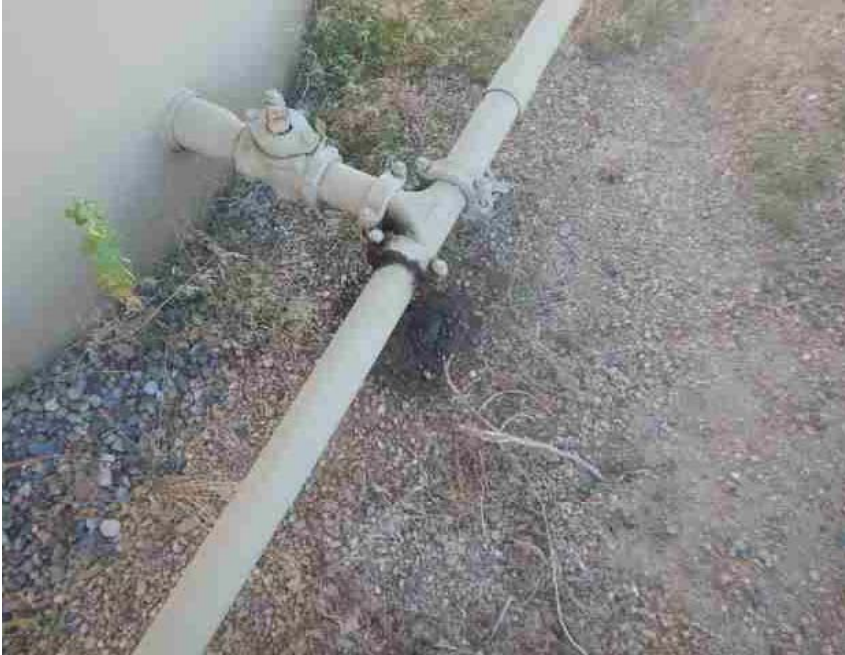
Prior inspection photo for comparison purposes only
