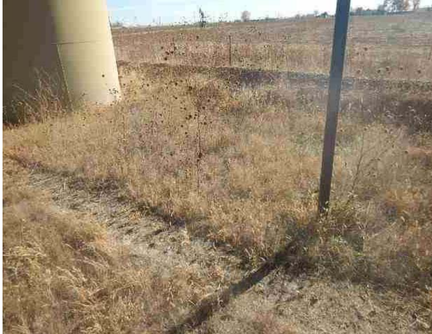
Prior inspection photo for comparison purposes only
