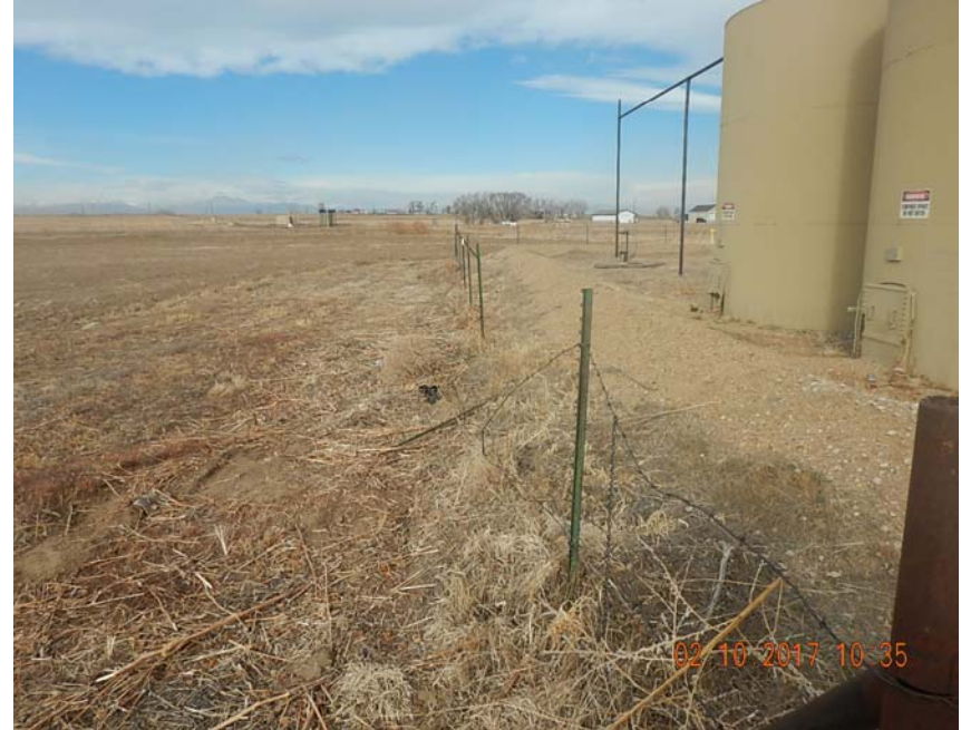
Photo 9: Tank battery fence in disrepair
