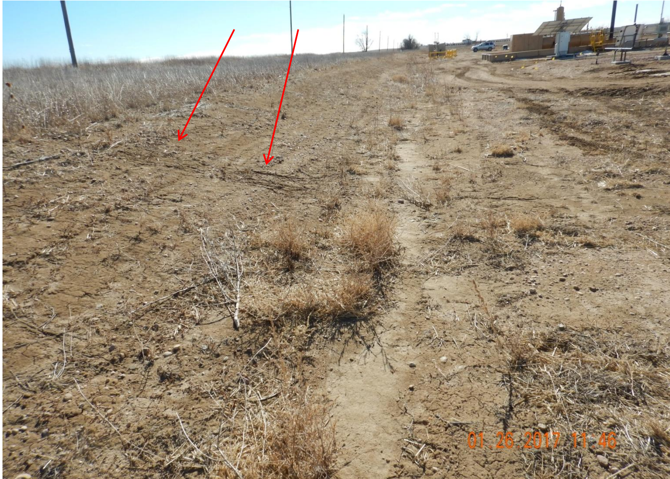
Photo 9. Photo taken from the eastern location, facing South. May need to monitor cut slope for erosion as it appears rill erosion is starting to form.
