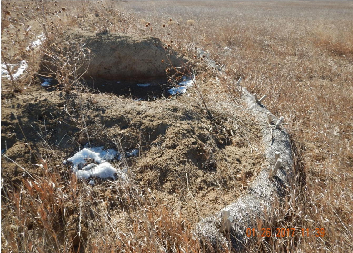
Photo 7. Photo taken from the northern sediment trap along the northwest location, facing South. Sediment was observed outside of containment area beyond the wattle.
