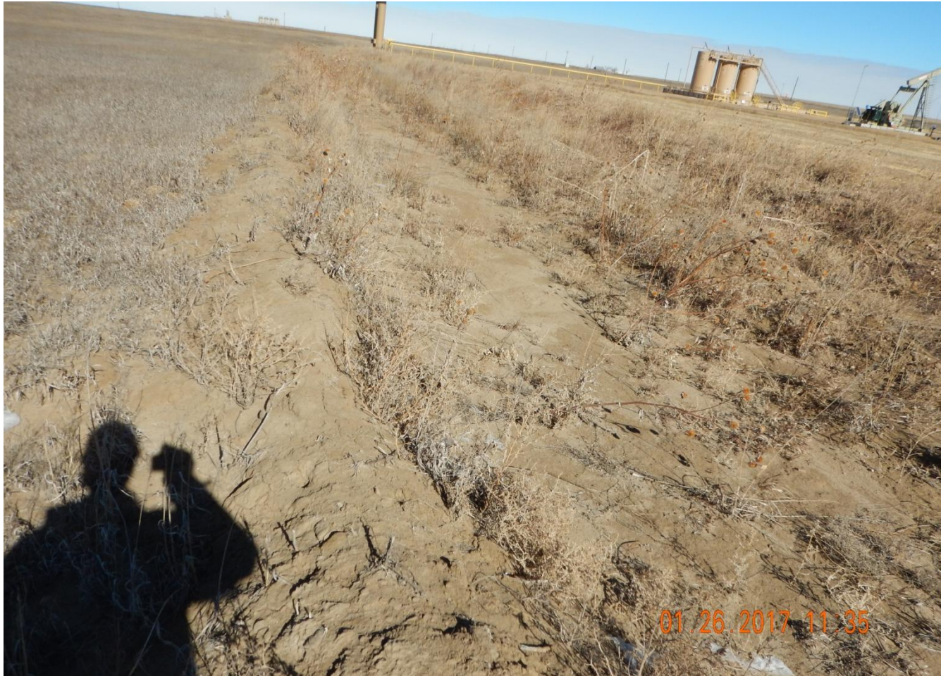
Photo 4. Photo taken from the southwest corner of location, facing North. Appears a retention area was constructed along the western location. The outer berm does not appear to be compacted and active erosion is occurring.
