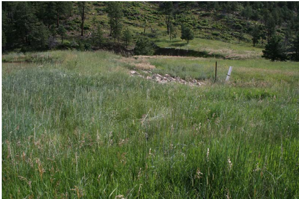
Photograph 2. Pond D, facing northeast across dam face from southwest end of dam.
