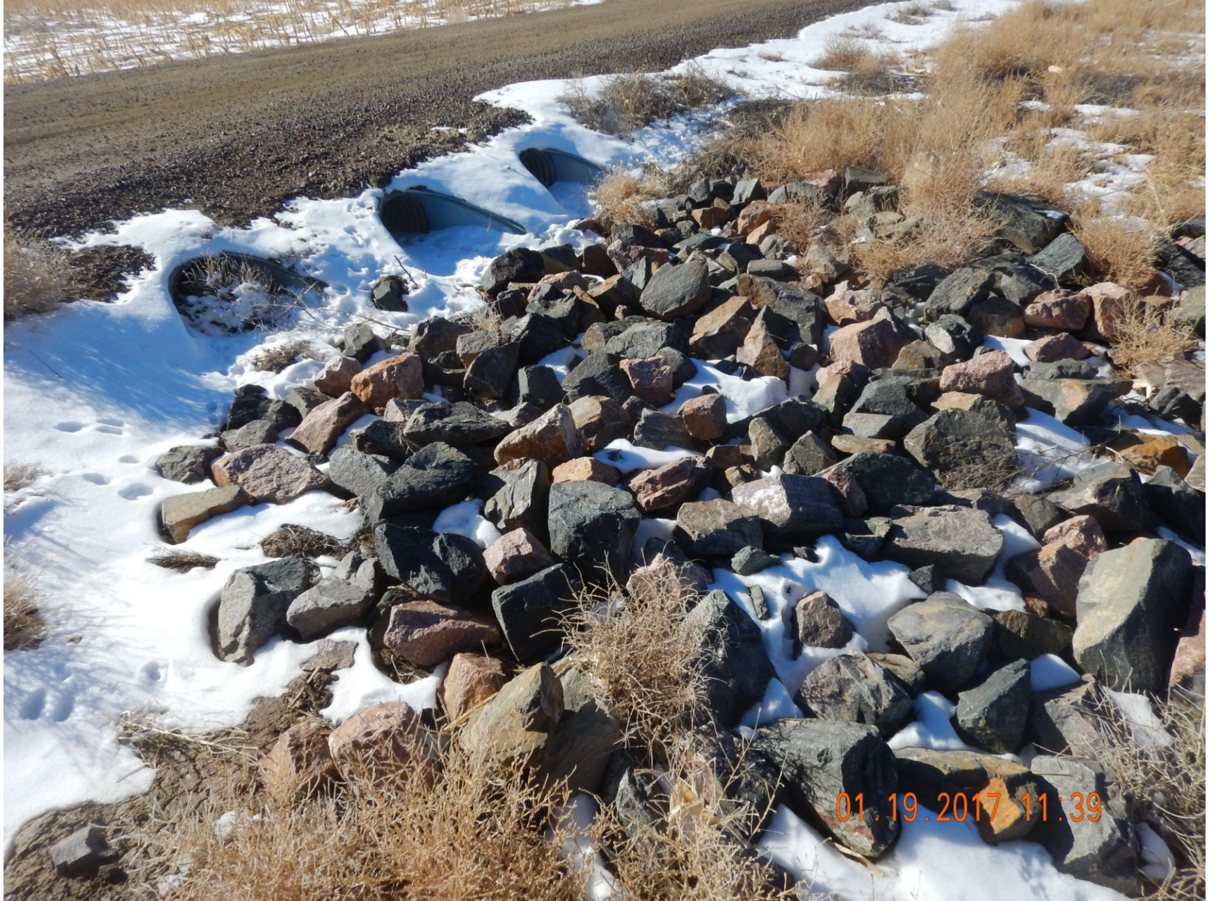
Figure 20: Photo taken from the access road near the country road, east .Photo shows culvert and stormwater BMPs
