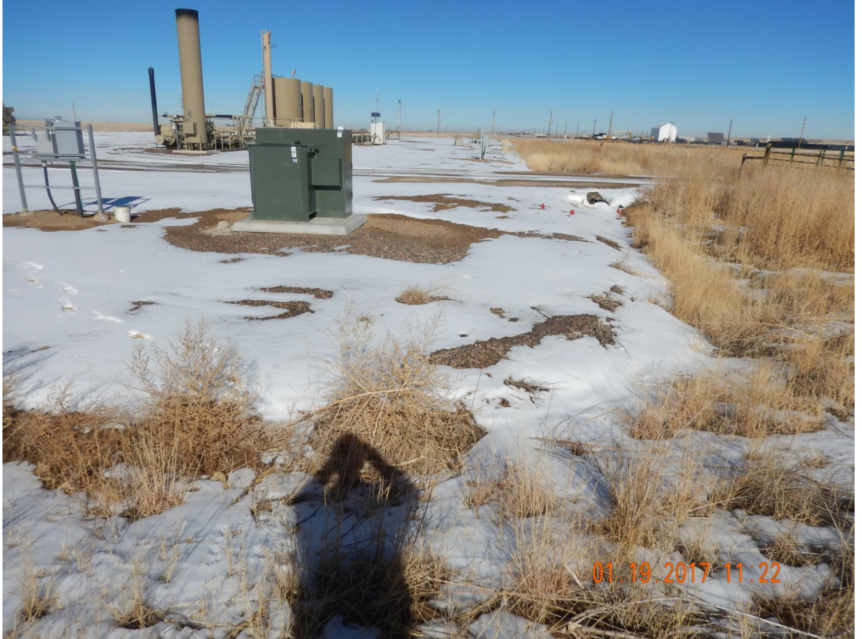
Figure 2: Photo taken from the southeast end of the location, facing north. Photo production and interim areas.
