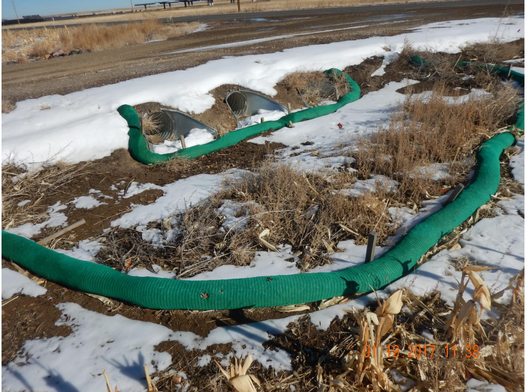
Figure 19: Photo taken from the access road near the country road, east .Photo shows culvert and stormwater BMPs
