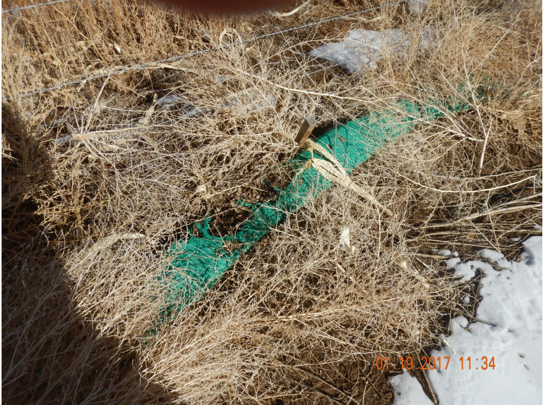
Figure 14: Photo taken from the northeast end of the location, next to sediment trap. Photo shows wattles used as stormwater and sediment control BMPs no longer in proper functioning condition.
