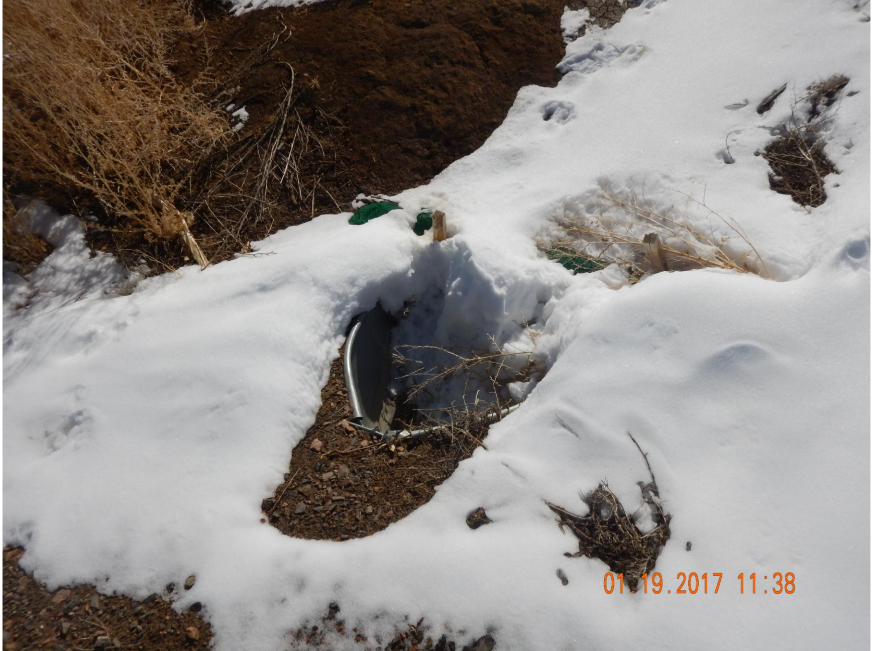
Figure 18: Photo taken from the east end of the location at access road. Photo shows culvert
