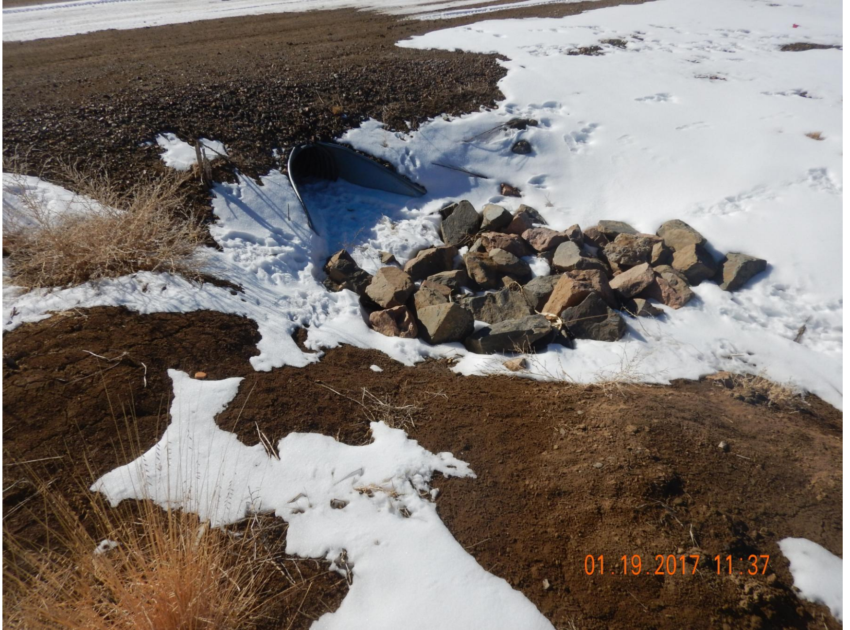
Figure 17: Photo taken from the east end of the location at access road. Photo shows culvert.
