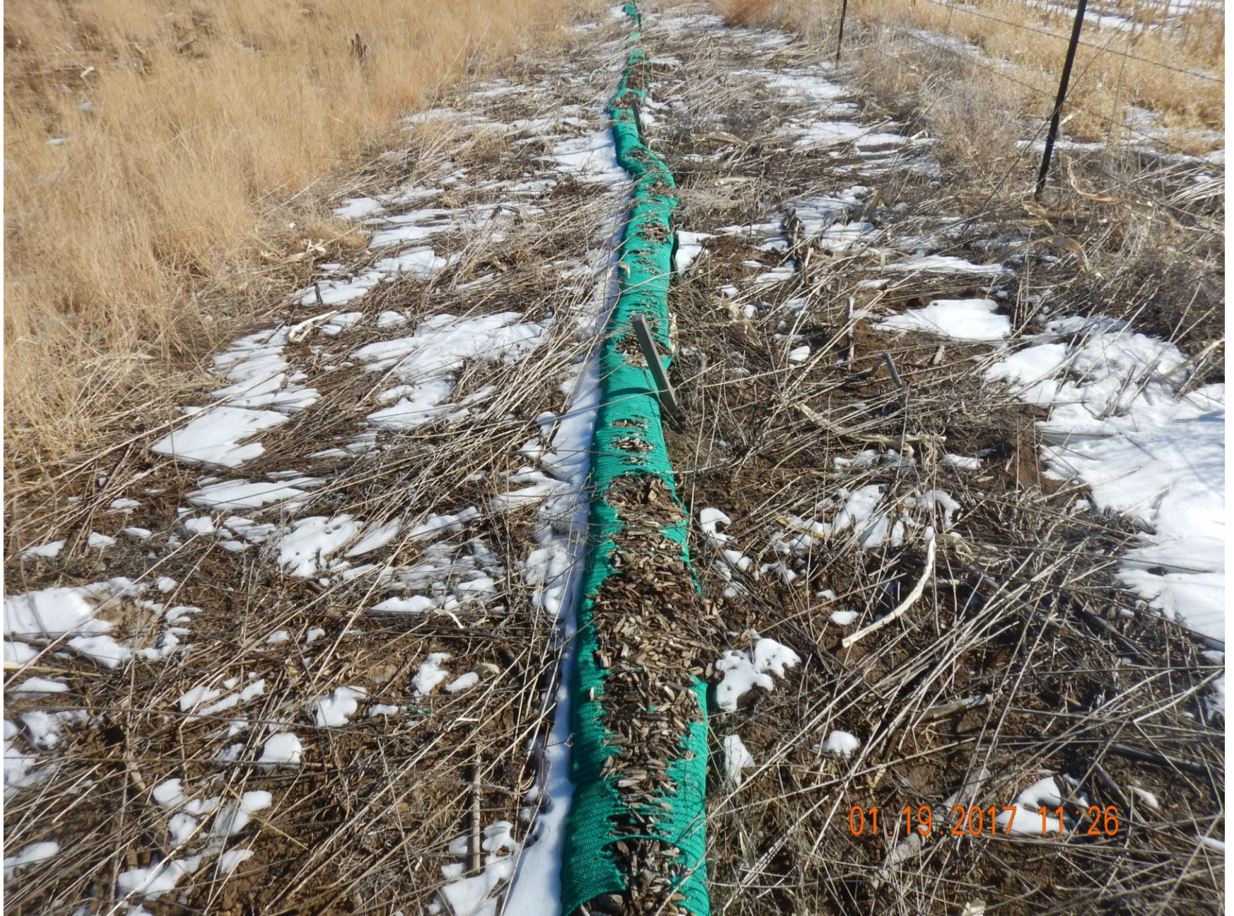
Figure 5: Photo taken from the south end of the location. Photo shows wattles used as stormwater and sediment control BMPs no longer in proper functioning condition.
