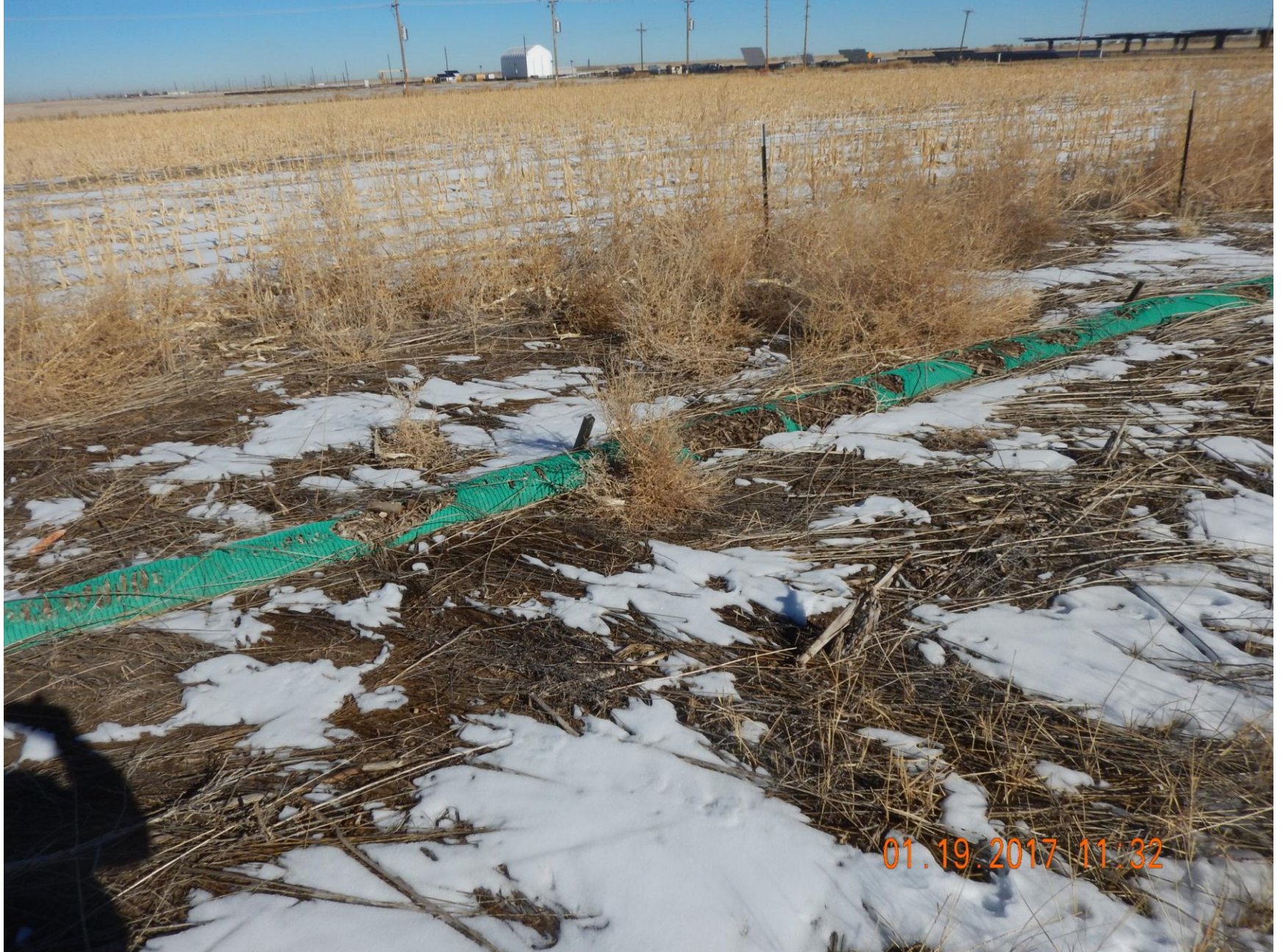
Figure 12: Photo taken from the north end of the location. Photo shows wattles used as stormwater and sediment control BMPs no longer in proper functioning condition.
