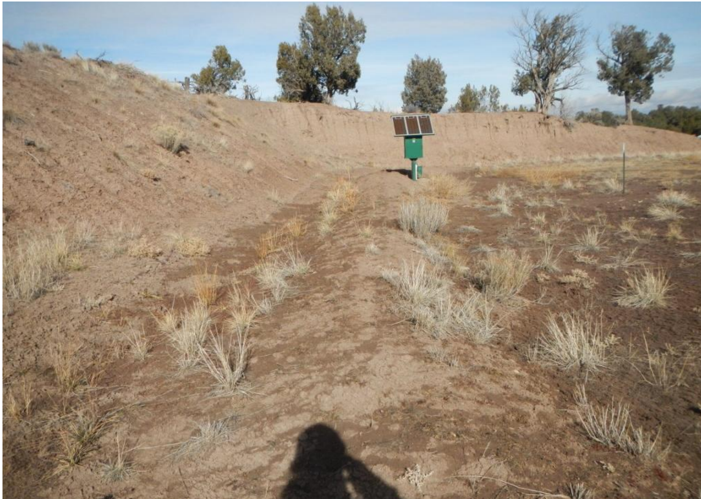
Photo 2. View of the western portion of the project area from the southwestern corner facing northward. Revegetation is sparse on cut-slopes and dominated by rubber rabbitbrush ( Chrysothamnus nauseosus ).
