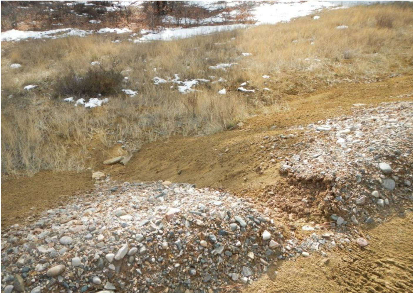
Photo 5. View of area in the southern portion of the project area where it appears stormwater has breached the stormwater berm. This area needs to be stabilized.
