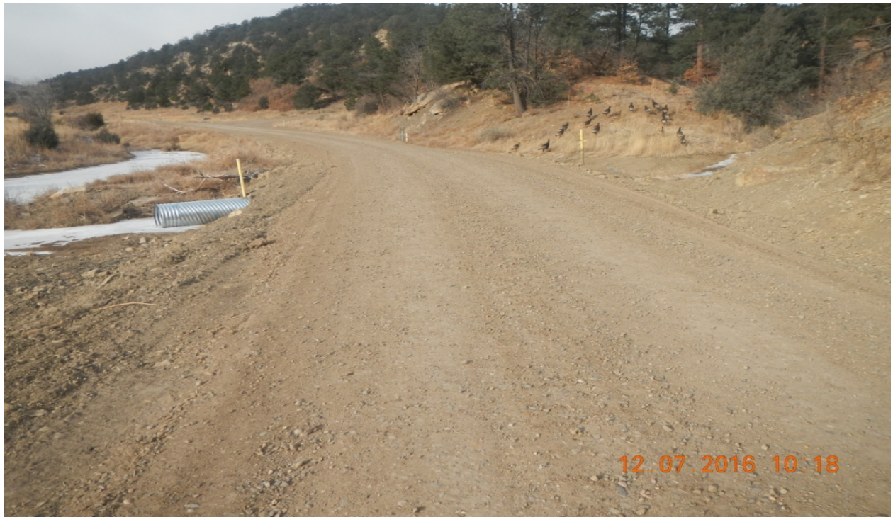
photo 1: Facing west along the main access road. A new culvert has been installed along the road and gravel has been applied.
