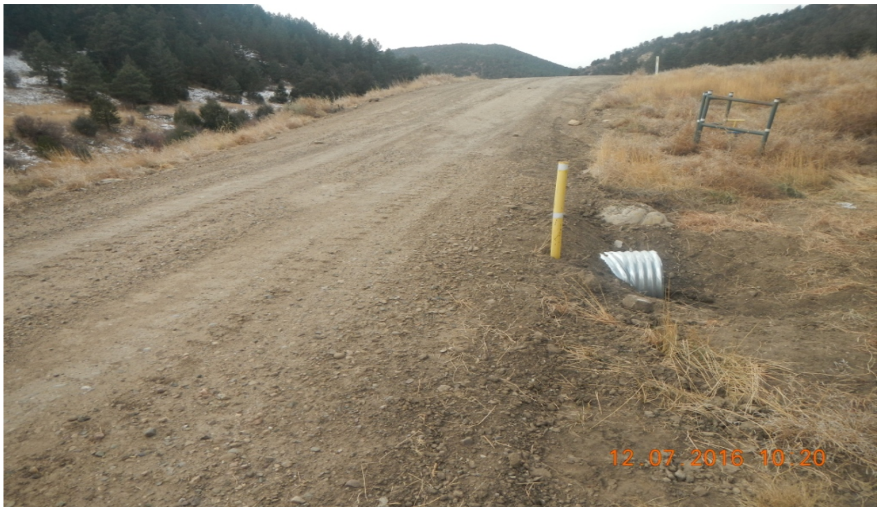
photo 2: Facing west along the main access road. A new culvert has been installed along the road and gravel has been applied.
