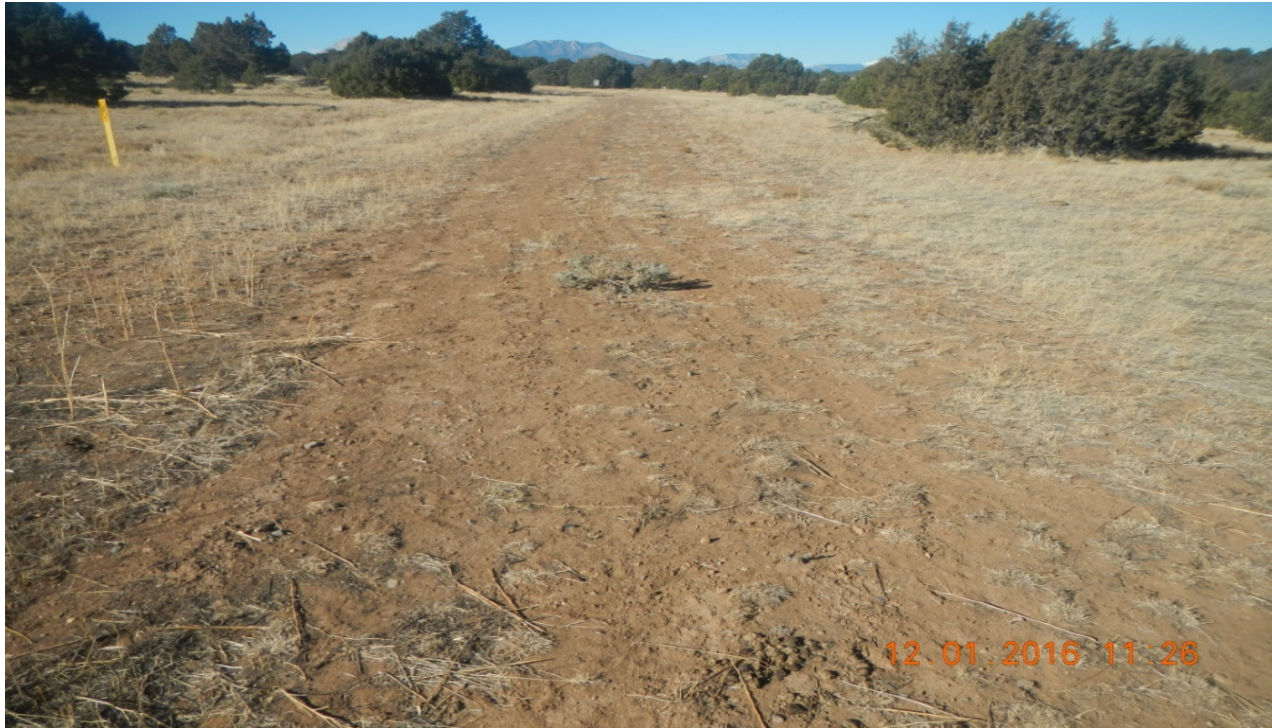
photo 1: Facing west along the former access road. The vegetation has not adequately established.
