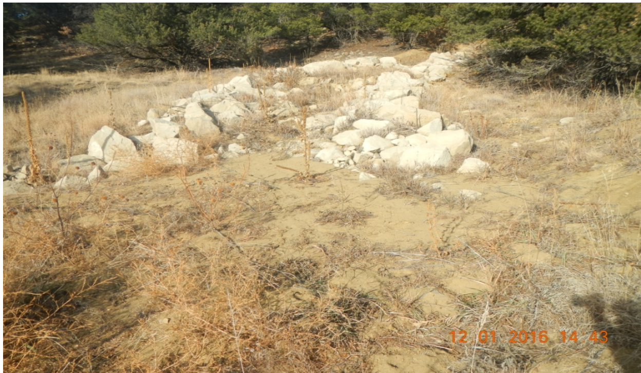
photo 4: A sediment trap along the western side of the location is filled in with sediment.
