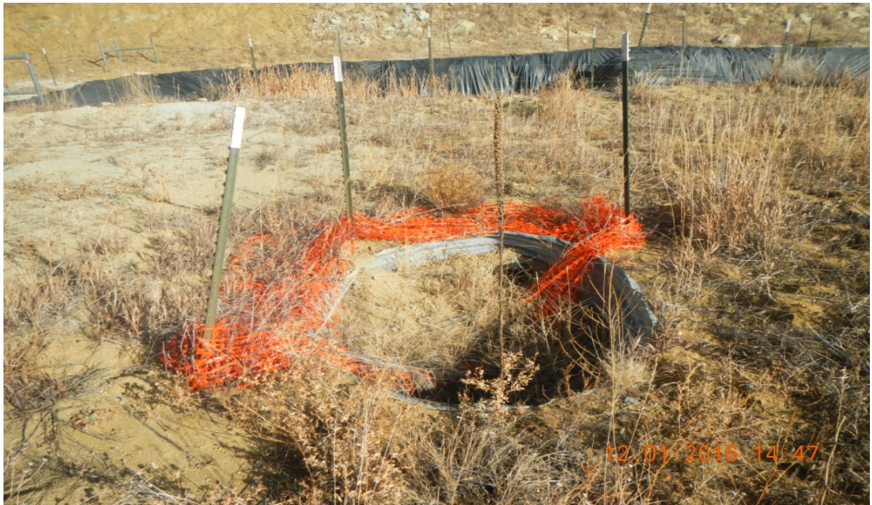
photo 11: Center of the location a conductor is present. Plastic safety fence is in disrepair.
