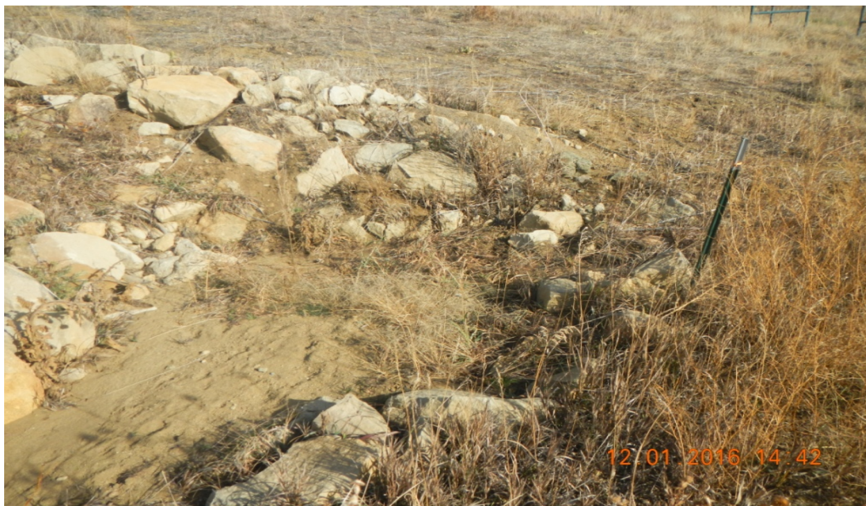
photo 3: The culvert near the access road is filled in with sediment.
