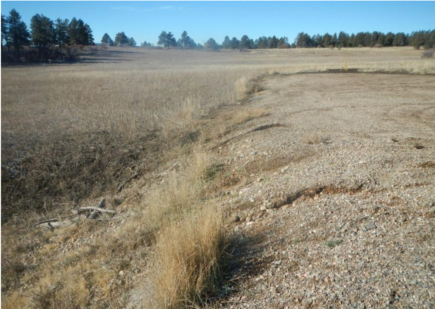
Photo 3. View of the southern portion of the project area from the southeastern corner facing westward. Rills on the edge need to be monitored and stormwater controls installed if it worsens.
