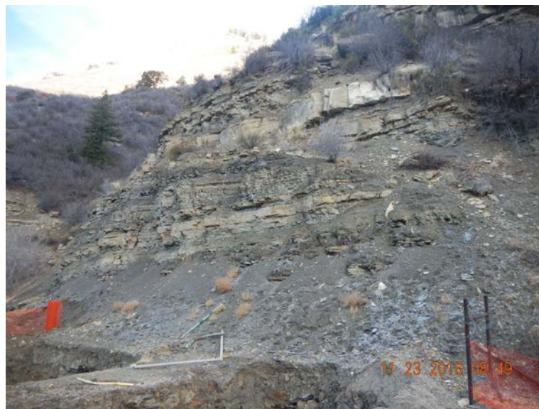
Steep unstable slope above excavation
