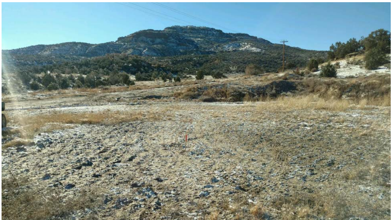
GREENLEAF DISPOSAL 1 PAD, NESW, SECTION 36, T 9 S, R 97 W, MESA COUNTY WELL PAD LOOKING SOUTH
