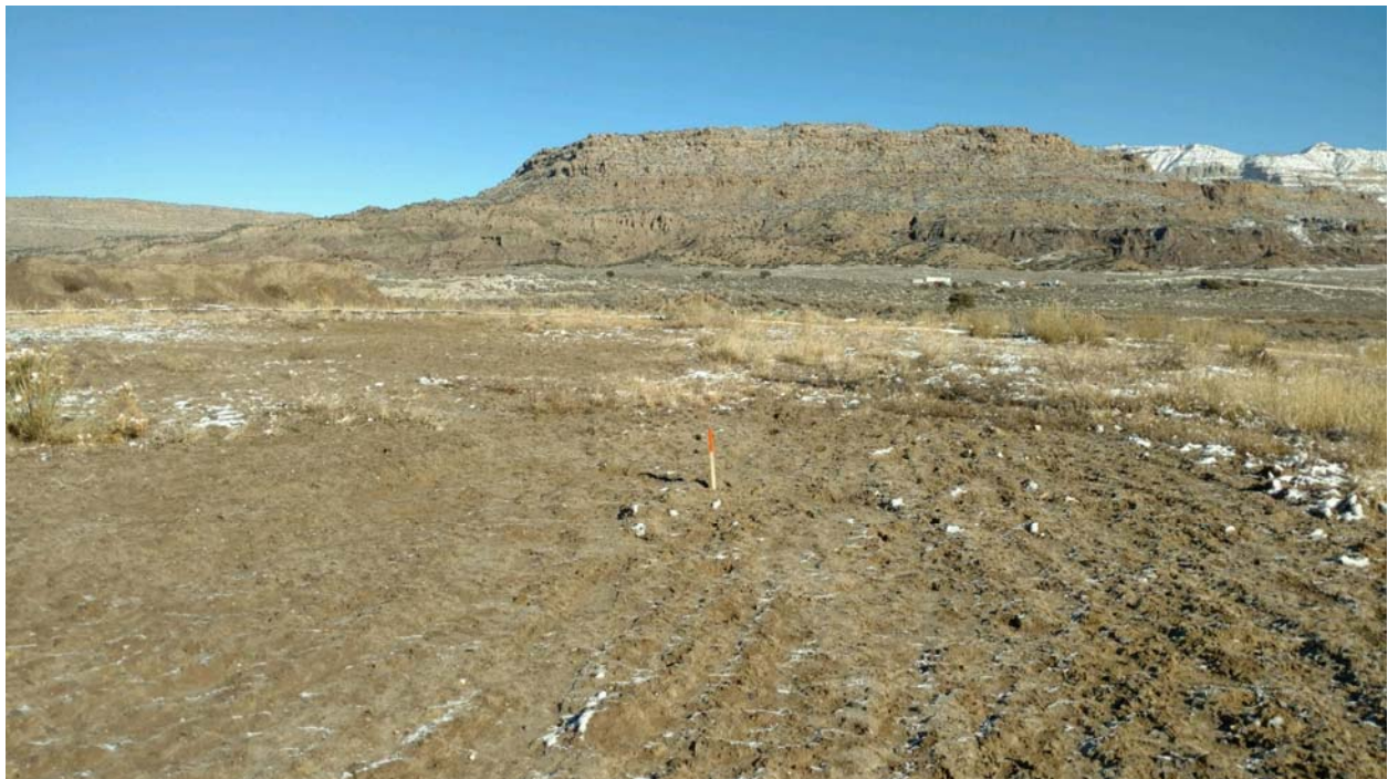
GREENLEAF DISPOSAL 1 PAD, NESW, SECTION 36, T 9 S, R 97 W, MESA COUNTY WELL PAD LOOKING NORTH
