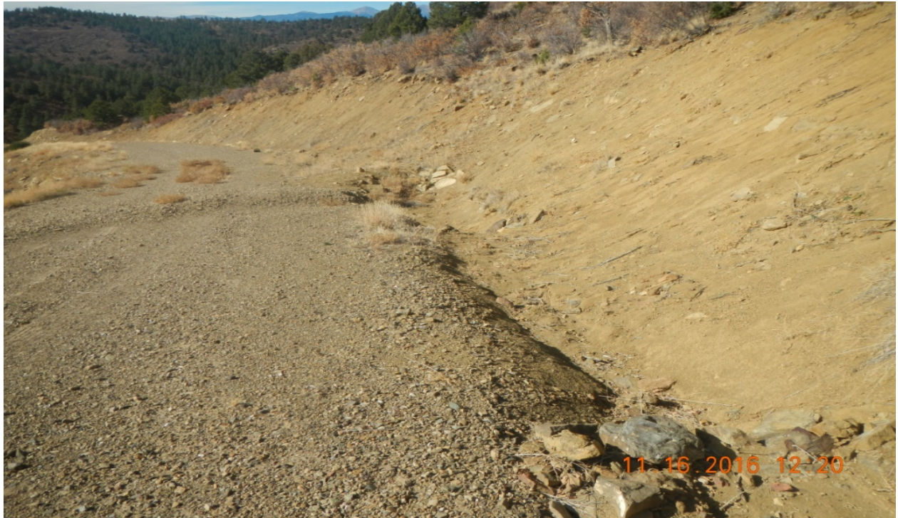
photo 3: The cut slope of the access road does not have much vegetation establishment for stabilization.
