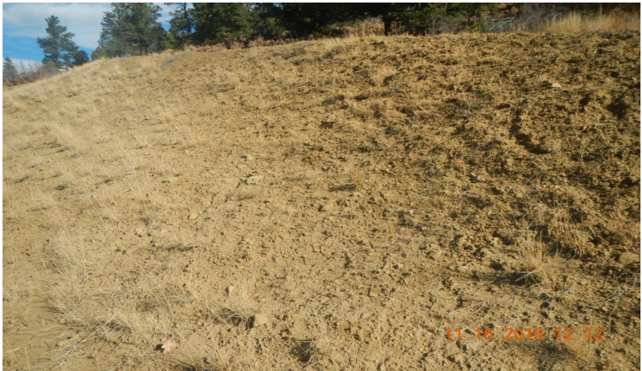
photo 10: The vegetation along areas of the cut slope does not appear to be adequately established.
