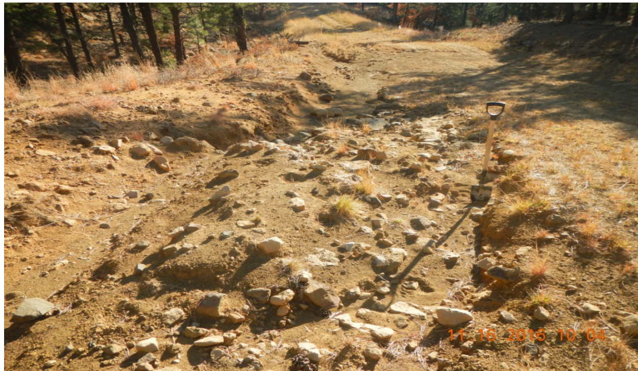
photo 4: Facing back to the east along the access road. There are signs of erosion occurring.
