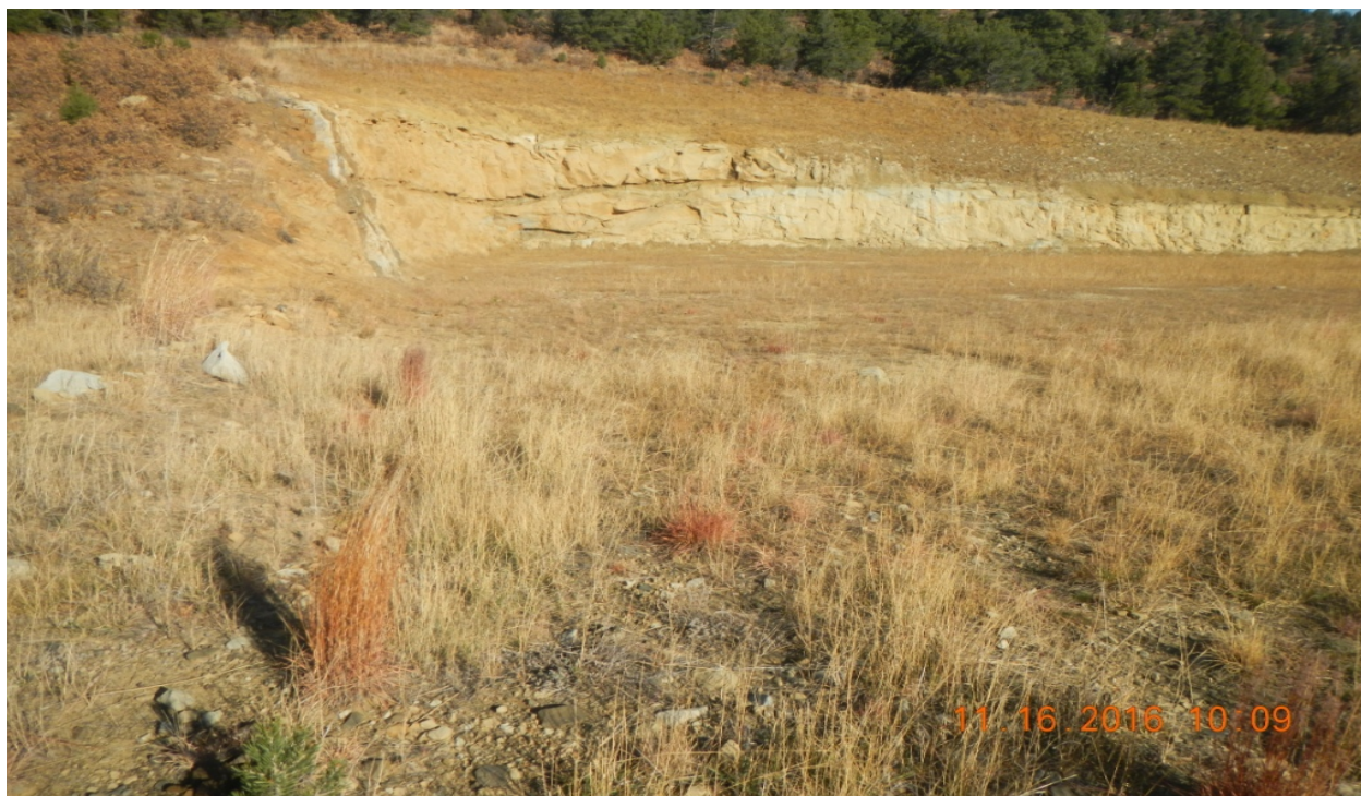
photo 13: East side of the location facing north toward the cut slope.
