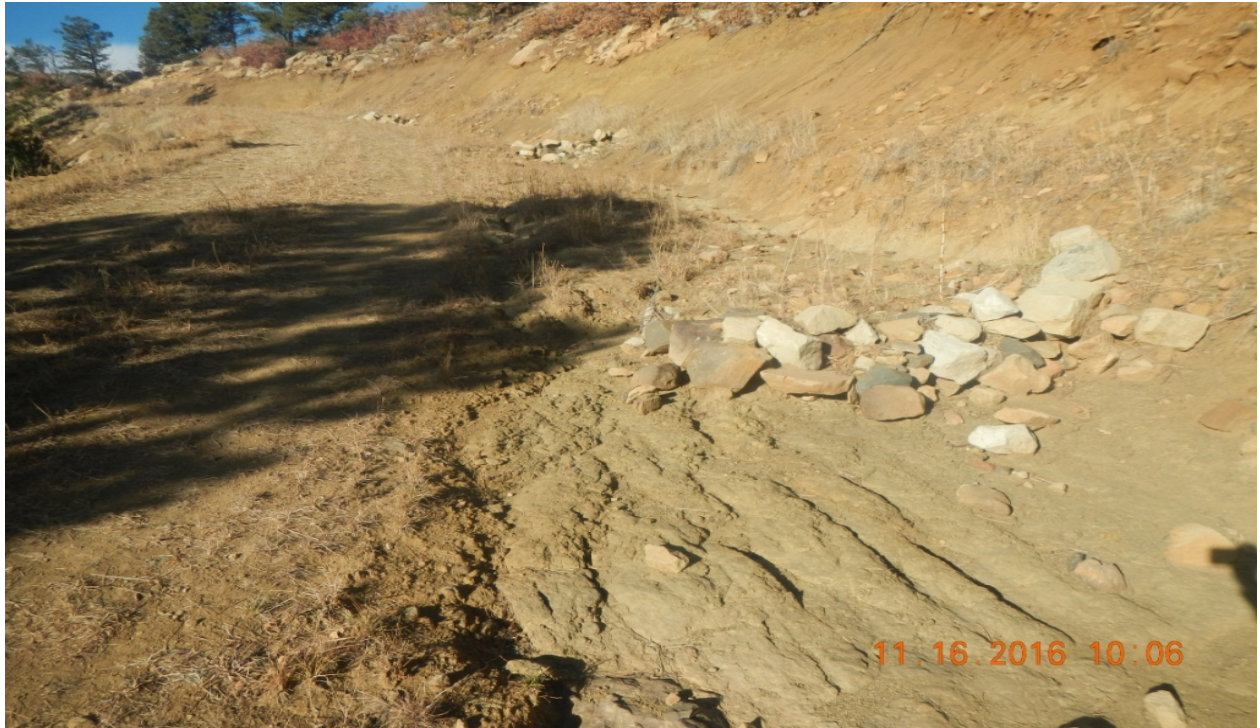
photo 7: Rock rip/rap has been placed at the north side of the location.
