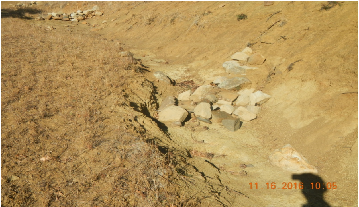
photo 5: The rock check dams are not maintained and erosion is occurring along the road side.
