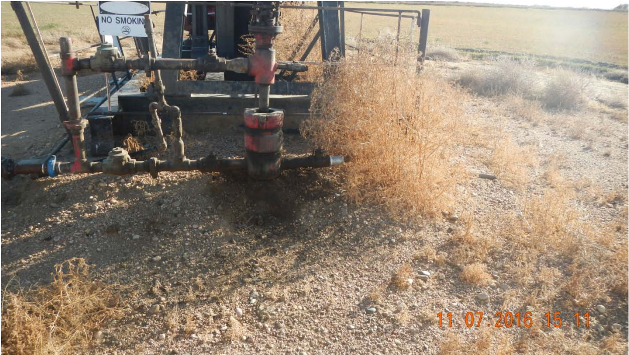
API # 123-09274, stained soil, debris.
