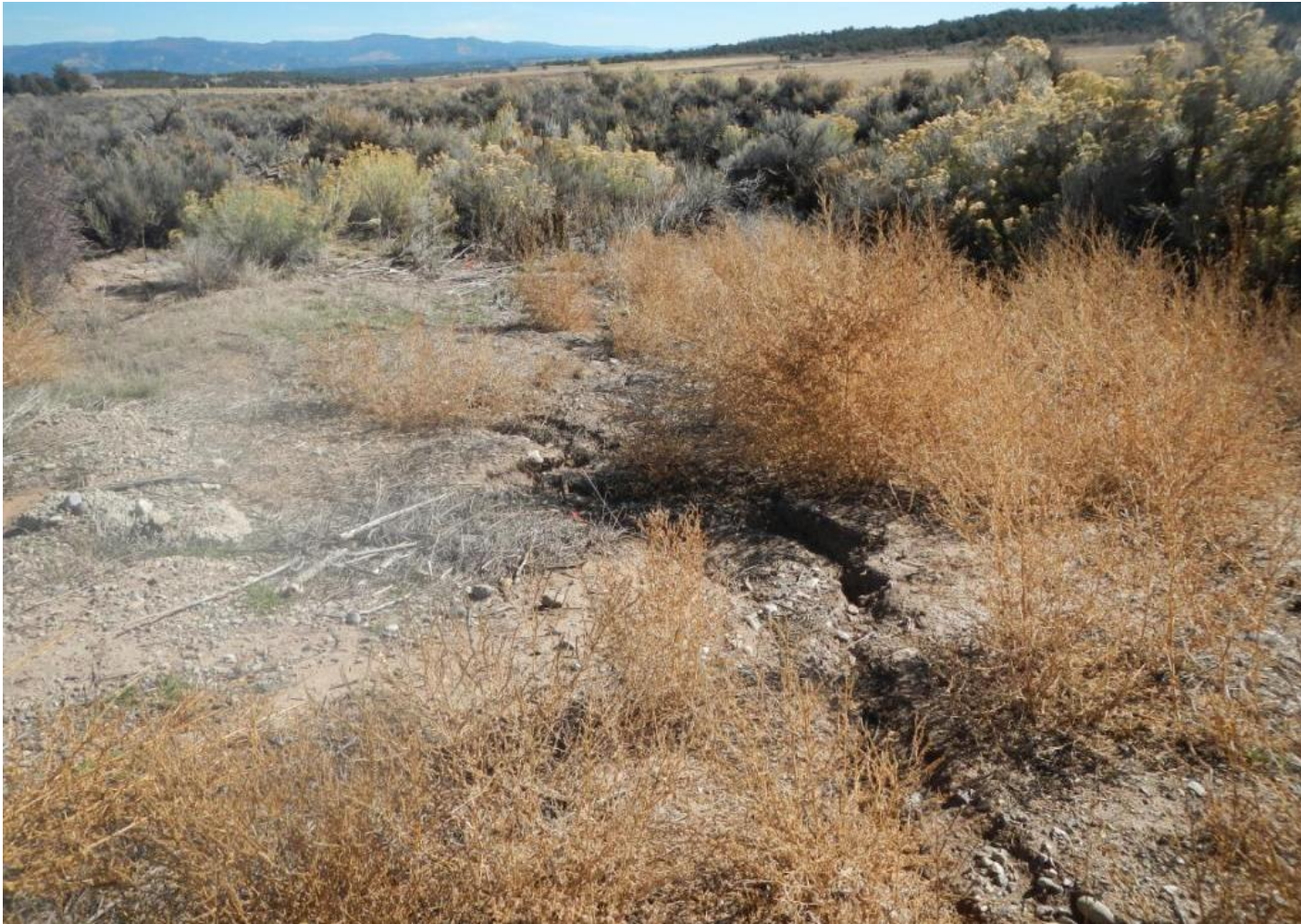
Photo 6. View of stormwater erosion and sediment deposition into a drainage in the northeastern corner of the project area.
