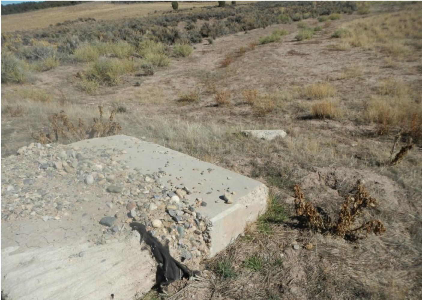
Photo 3. View of cement debris that needs to be removed in the eastern portion of the project area.
