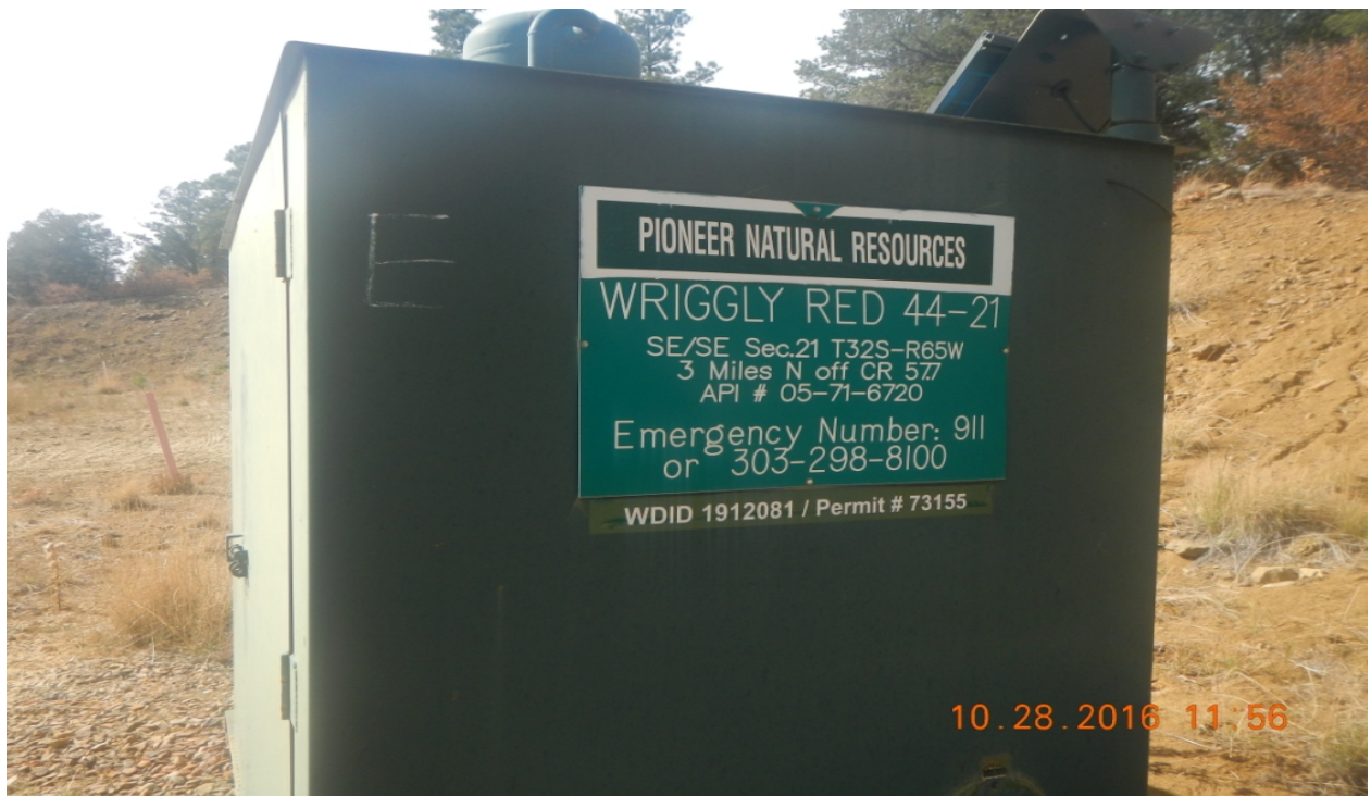
photo 2: Well sign. The emergency number is disconnected.
