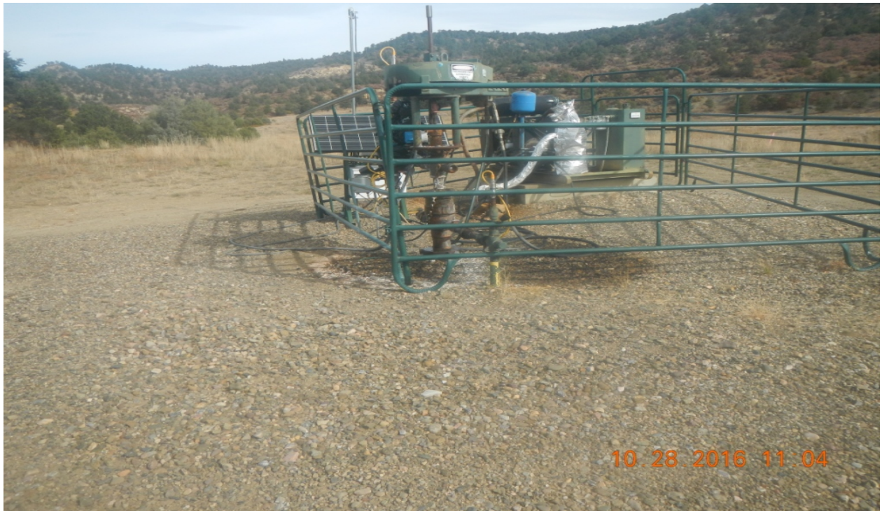
photo 1: Facing northeast toward the wellhead.
