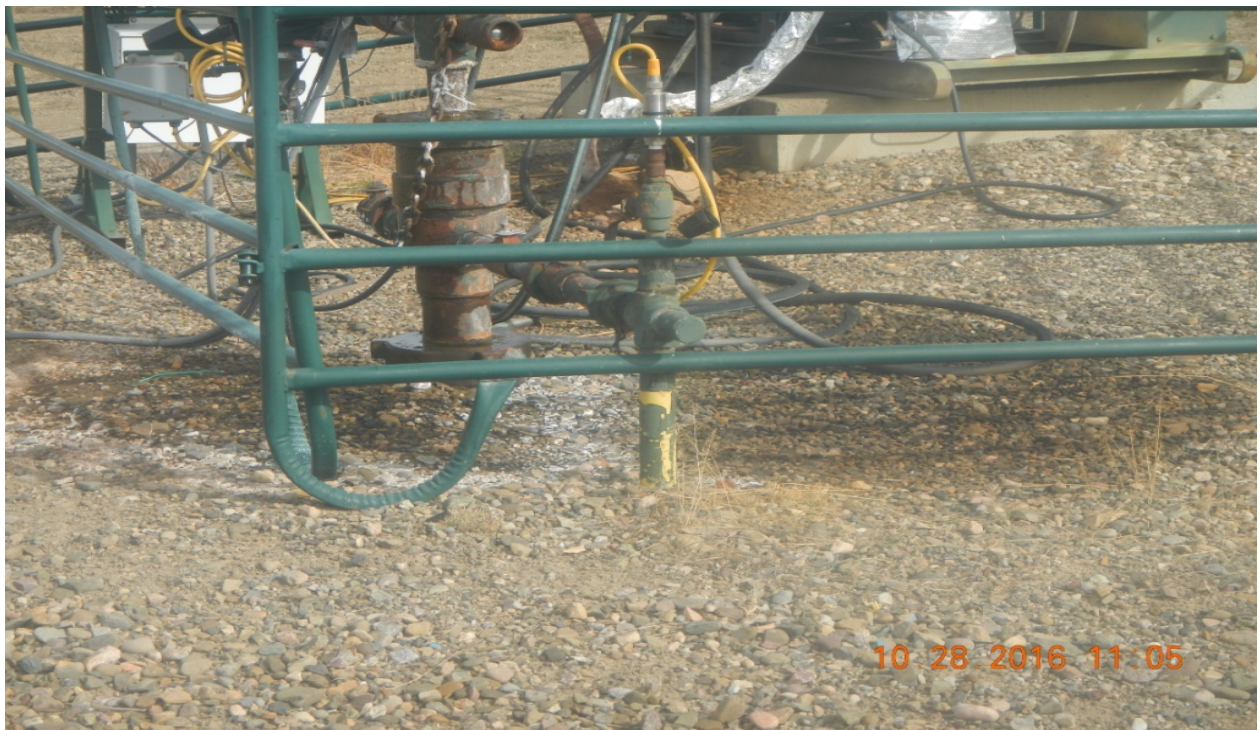
photo 2: There is a dripping water leak from the wellhead.
