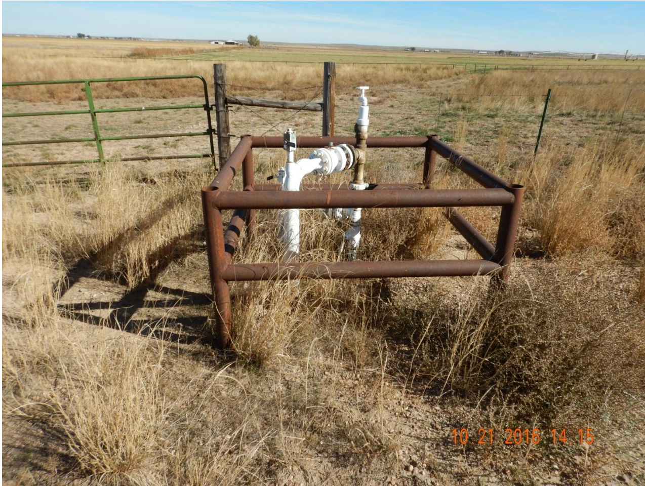
Photo 6. Photo taken from tank battery location, facing East. Need to remove pipeline risers per Rule 1004.
