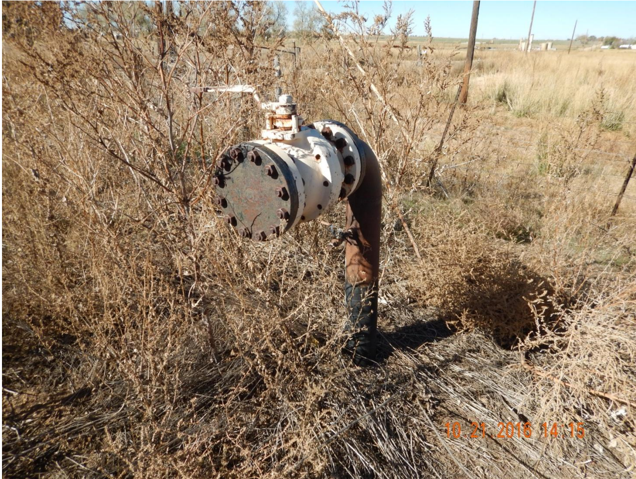
Photo 7. Photo taken from tank battery location, facing North. Need to remove pipeline risers per Rule 1004.
