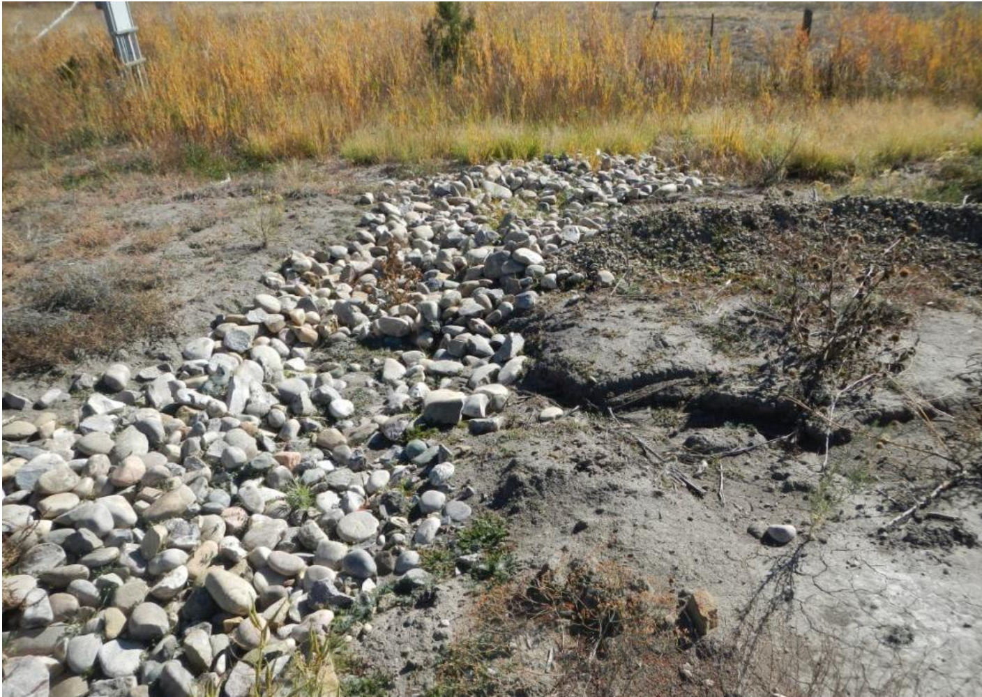
Photo 2. View of new cobble run-down in the northeastern corner of the project area.
