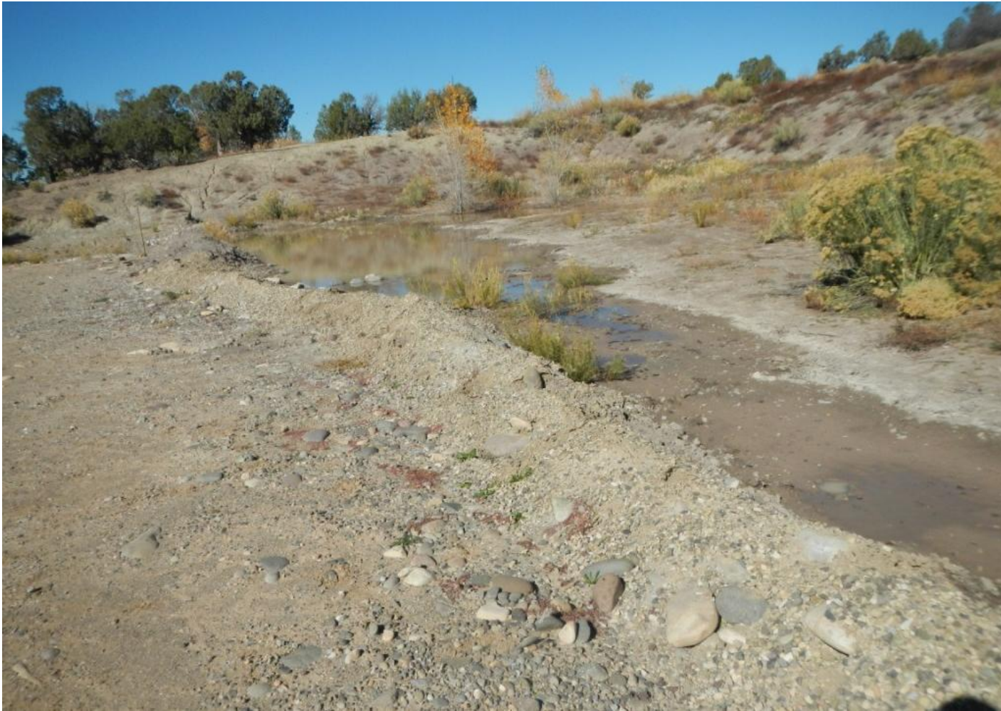
Photo 3. View of new berm on the northern edge of the working area, appears to be functioning.
