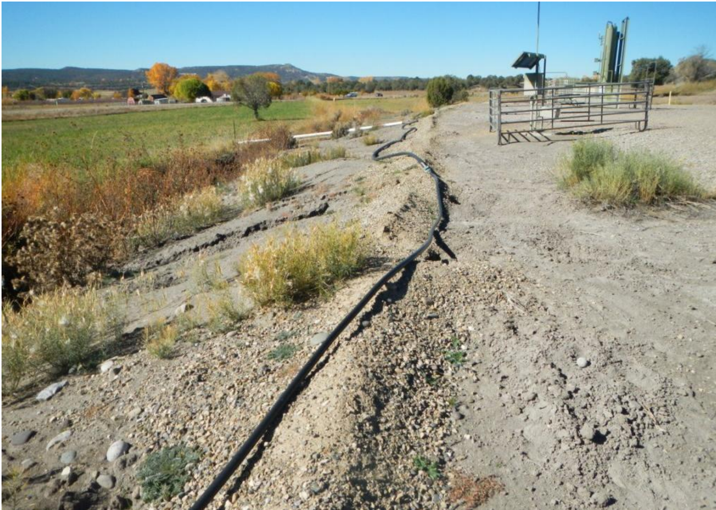
Photo 5. View of new berm along the southern edge of the working area. This berm is not sufficient at controlling stormwater erosion along the southern fill slope where significant erosion is occurring from exposed soils eroding into adjacent irrigation ditch.
