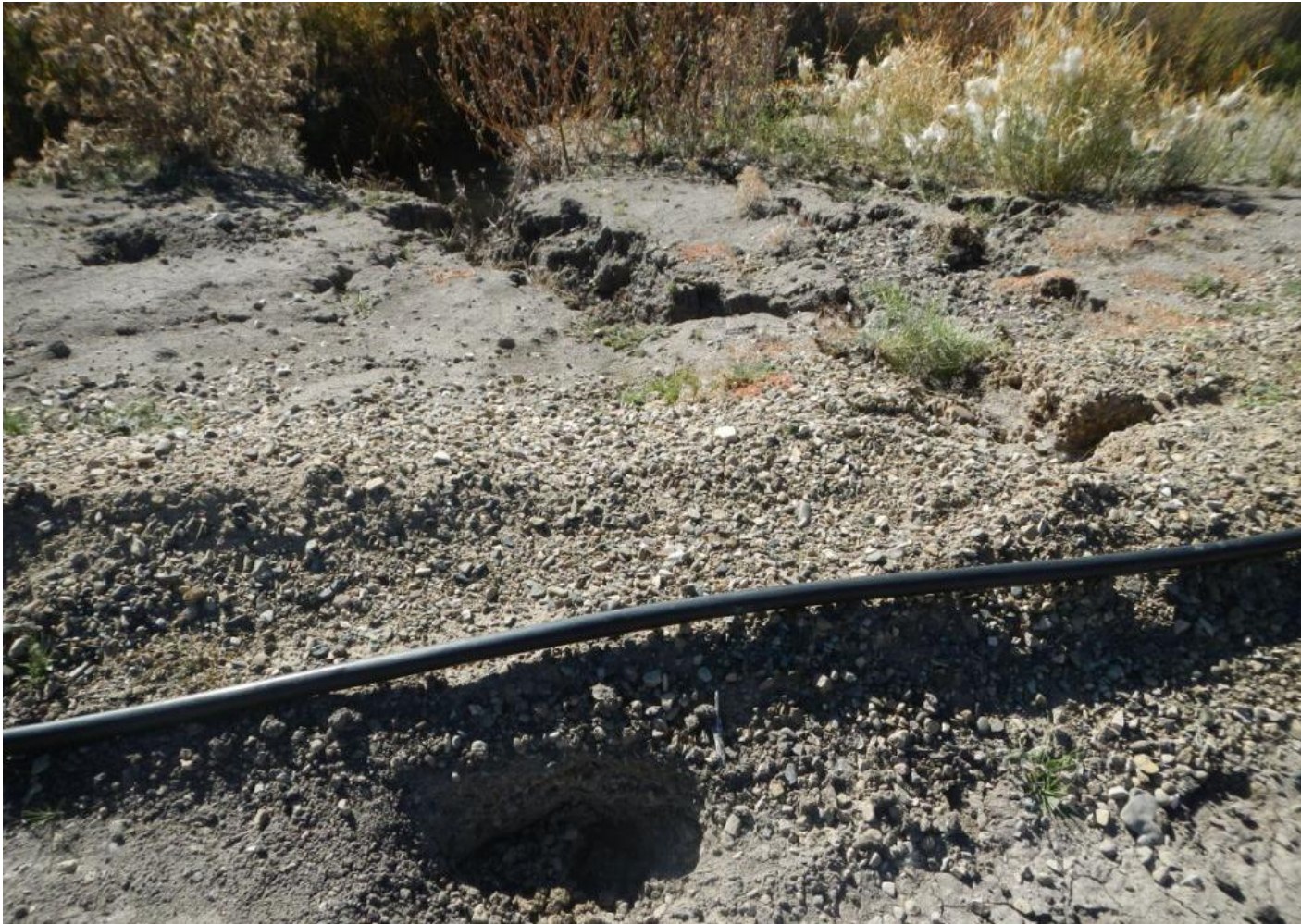
Photo 7. Another area along southern edge where berm is eroding (facing downslope).
