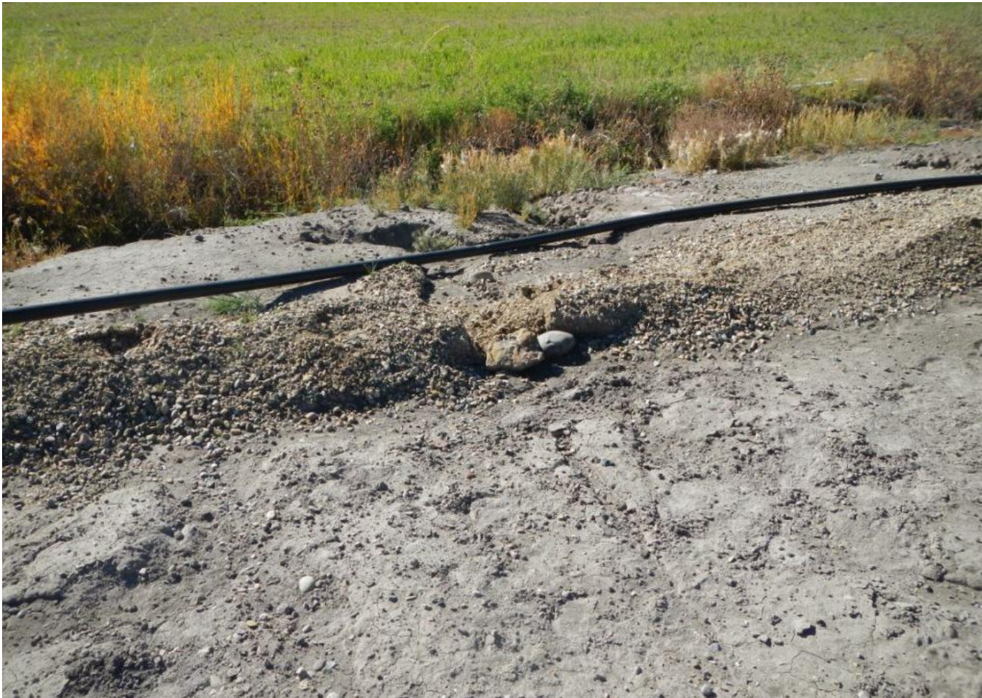
Photo 6. View of area on southern edge of well pad where new berm is eroding (facing downslope toward ditch).
