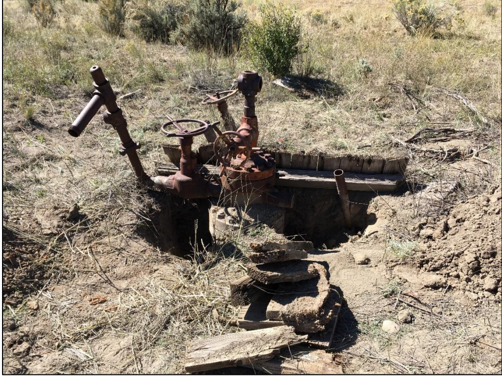
Photo 1: McCulloch #4 Well Head
