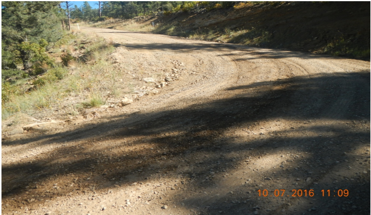
photo 5: The main road switches back to the northeast at this point. Erosion issues have been corrected.
