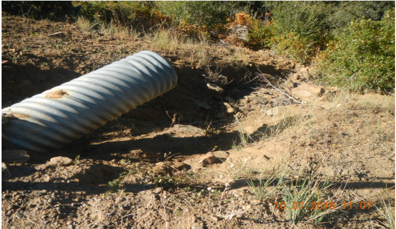
photo 3: It was noticed that some culverts do not have outlet protection which is a potential for erosion.
