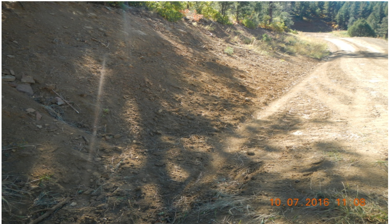
photo 4: The side of the access road was reggraded and seeded. Stormwater is now properly diverted.
