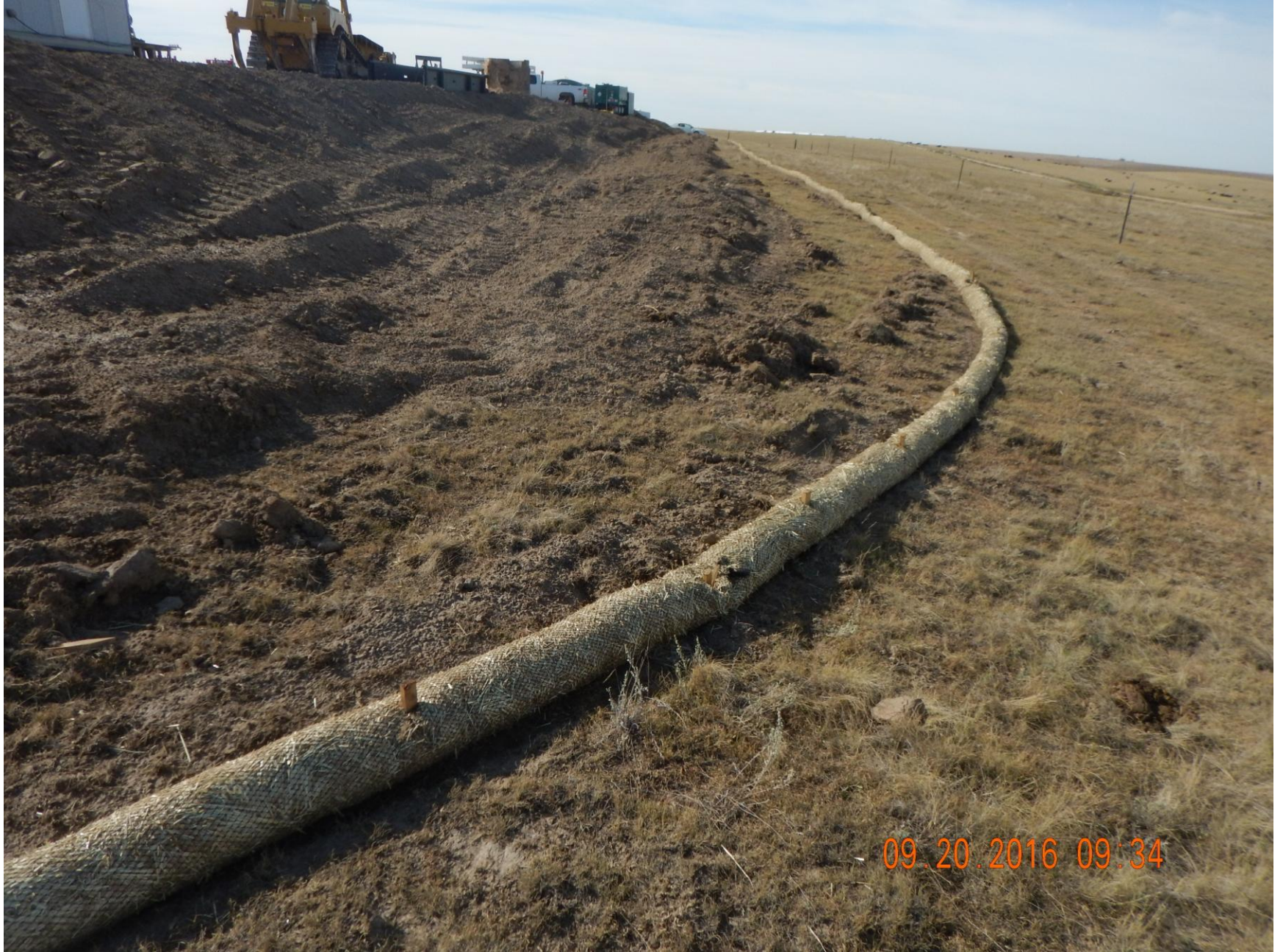
Figure 2: Photo taken from the northwest corner of the location, facing south. Photo shows straw wattles used as stormwater and sediment control BMPs have been properly entrenched.
