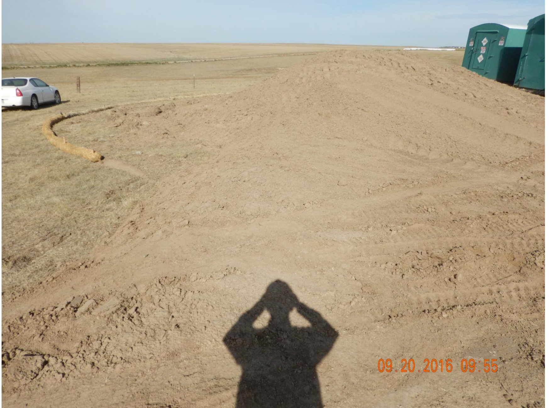
Figure 4: Photo taken from the southwest corner of the location. Photo shows topsoil pile. Construction foremen had mentioned they placed additional topsoil at this, and one other location to the southeast when they expanded the location.
