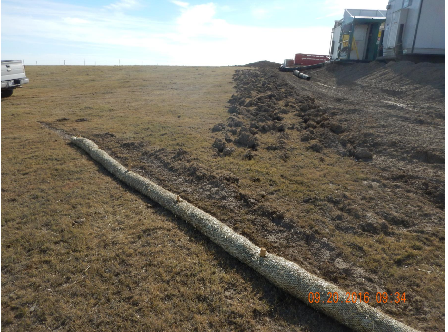
Figure 3: Photo taken from the northwest corner of the location, facing east. Photo shows straw wattle “j-hook” had been extended and additional surface roughening had been incorporated.
