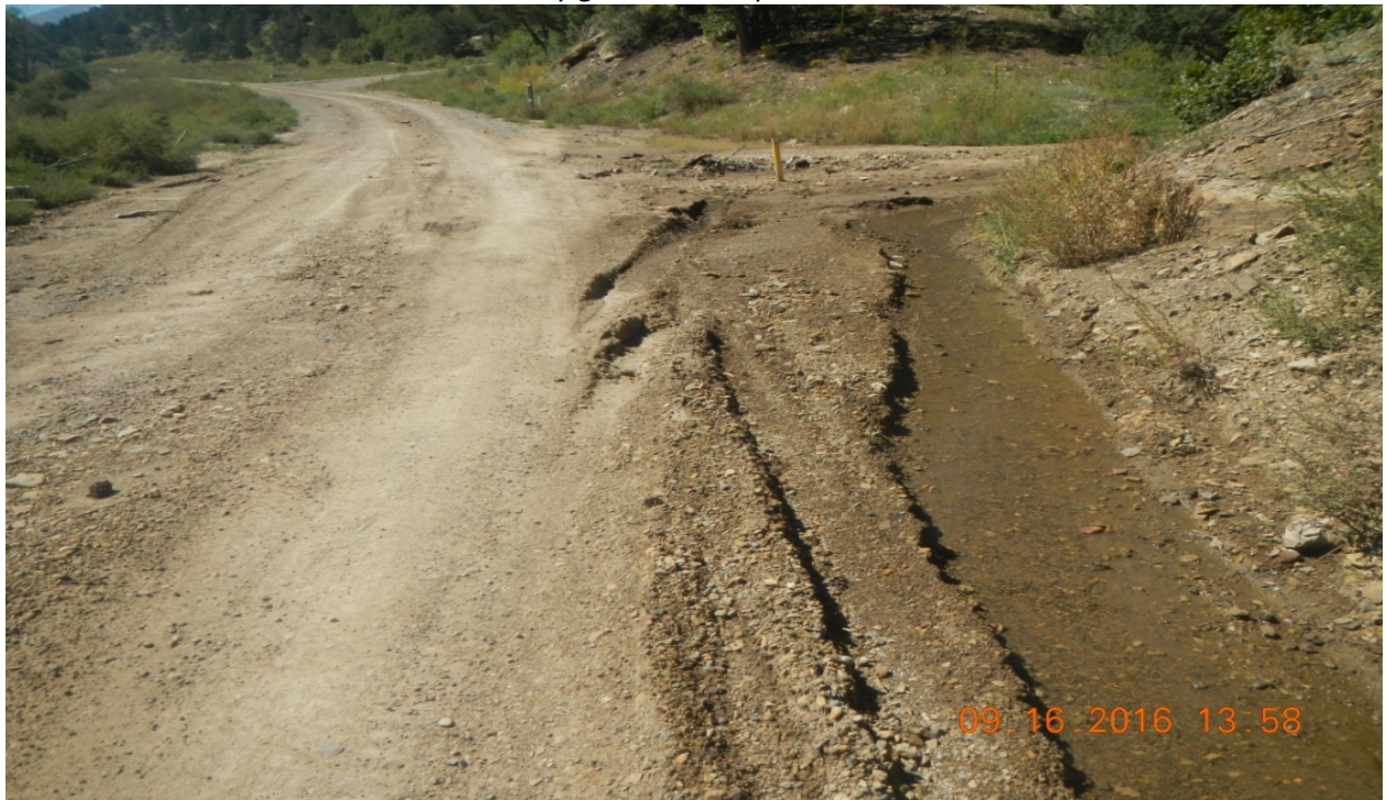
photo 2: Facing west along the main access road. Sediment has filled in the culverts. Stormwater flowed across the road which washed away gravel and deposited sediment on the road.
