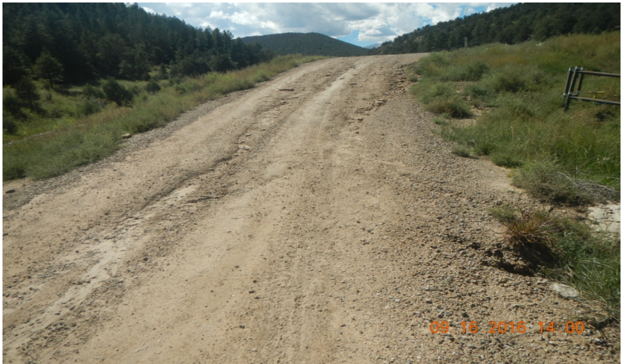
photo 4: Facing west along the main road near the location. There are signs of erosion occurring on the road.
