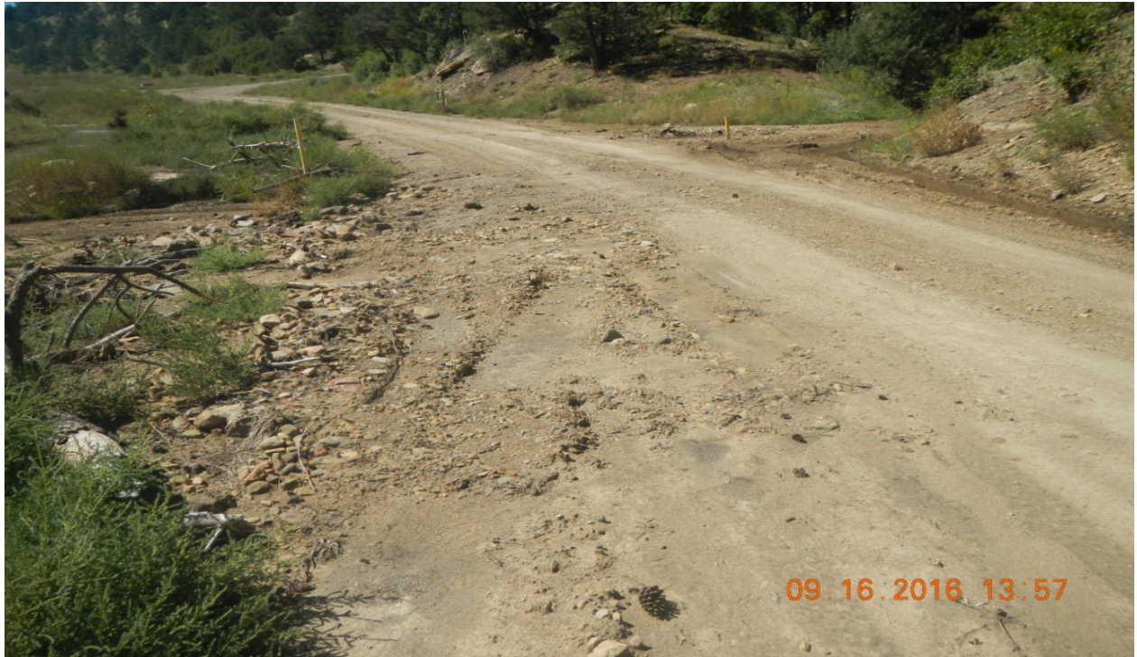
photo 1: Facing west along the main access road. Sediment has filled in the culverts. Stormwater flowed across the road which washed away gravel and deposited sediment on the road.
