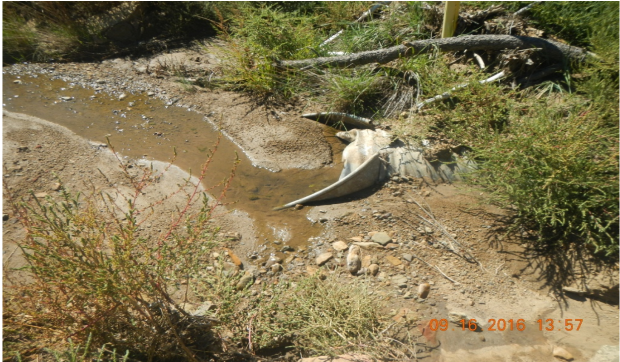
photo 3: The culvert along the main road has filled in with sediment.
