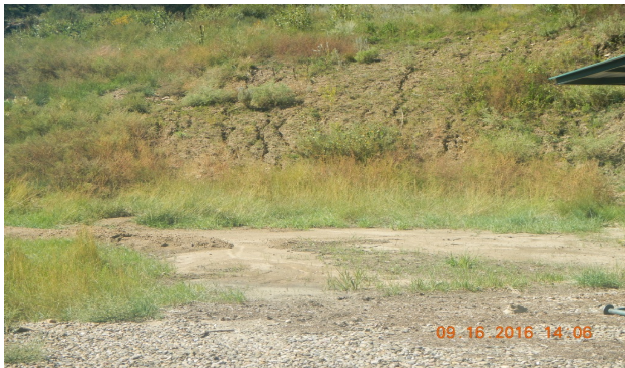
photo 5: Facing toward the northwest cut slope. There are signs of erosion in this area.
