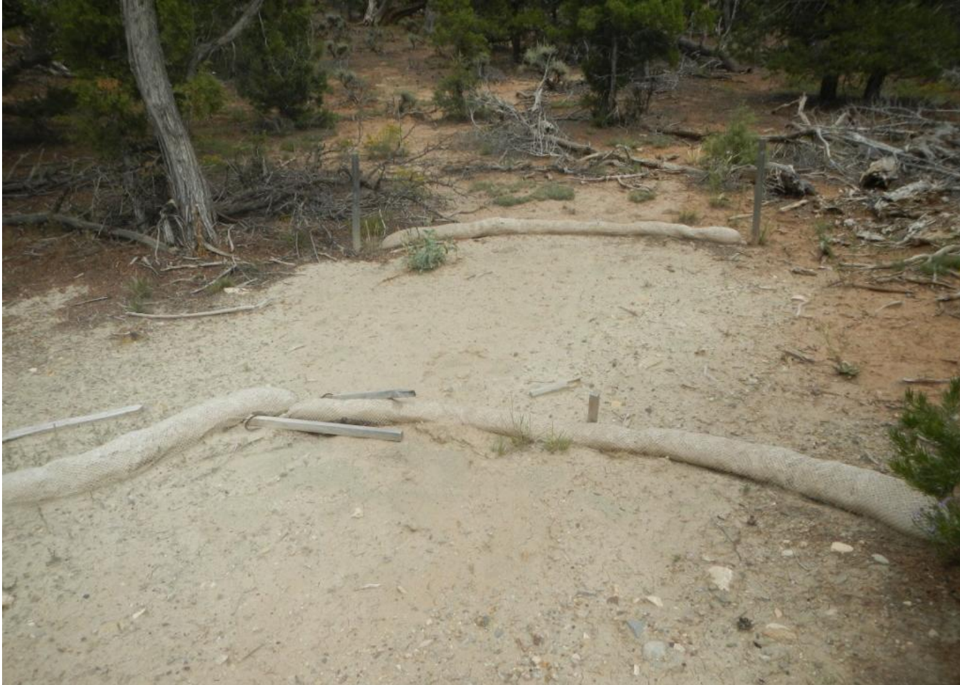
Photo 9. View of wattles in the northeastern corner of the well pad in disrepair.
