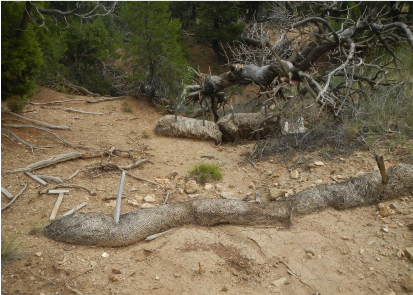
Photo 8. View of wattles and hay bales in the northwestern corner in disrepair.
