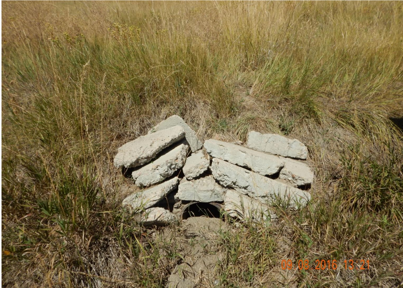
Photo 9. Photo taken of Culvert #2 that remains behind and needs to be removed.
