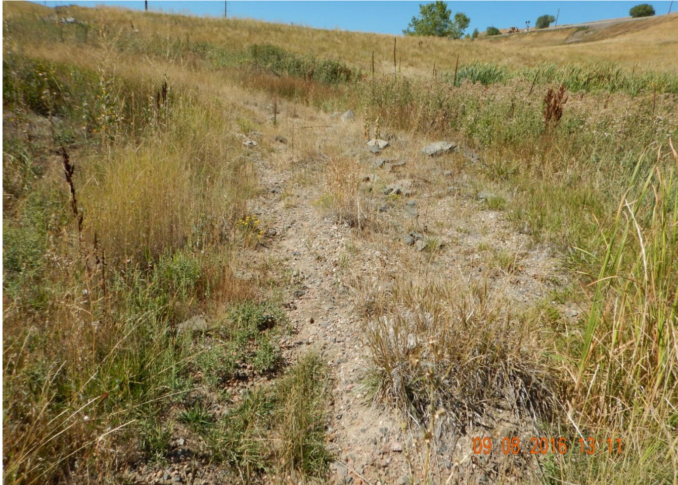
Photo 8. Photo taken from Culvert #1, facing West. Access road needs to be stabilized with native, perennial vegetation to prevent further erosion.
