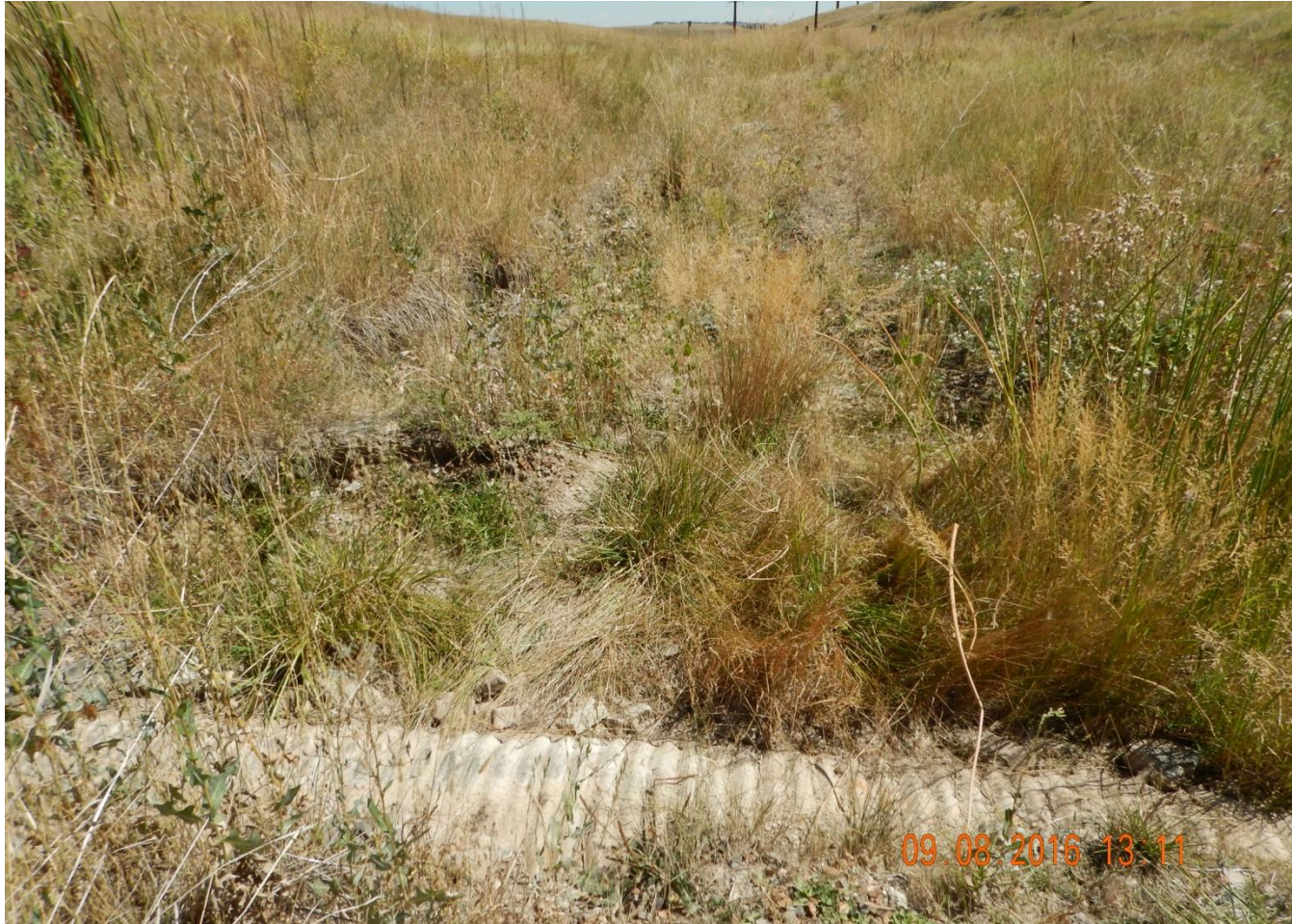
Photo 7. Photo taken from Culvert #1, facing East. Culvert needs to be removed to establish natural flows, need to remove gravel used to arm the culvert and reseed with native, perennial vegetation that is representative.
