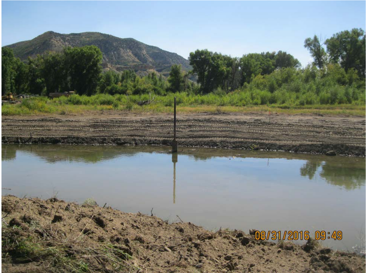
Williams Fork River channel has meandered exposing surface casing. No signs of leaks. Looking east.
