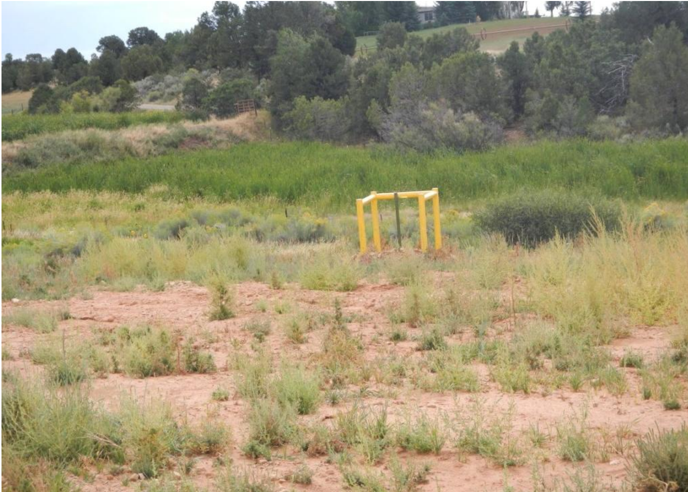
Photo 4. View of another riser that needs to be removed south of the project area.
