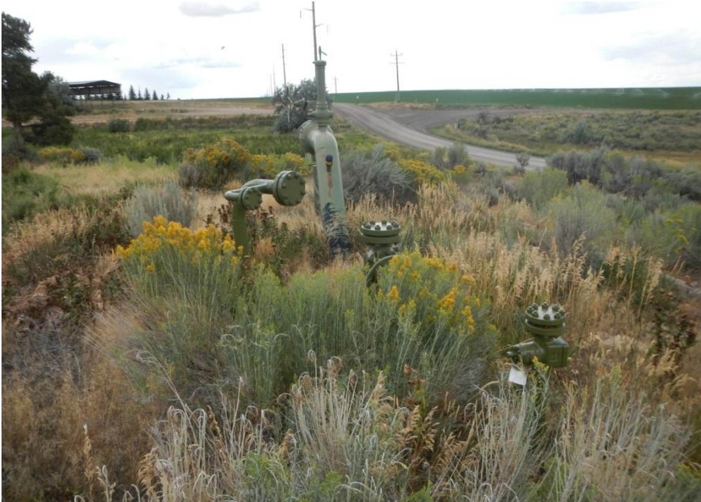
Photo 2. View of pipeline riser south of the access road that needs to be removed or documentation provided showing that it is in use.
