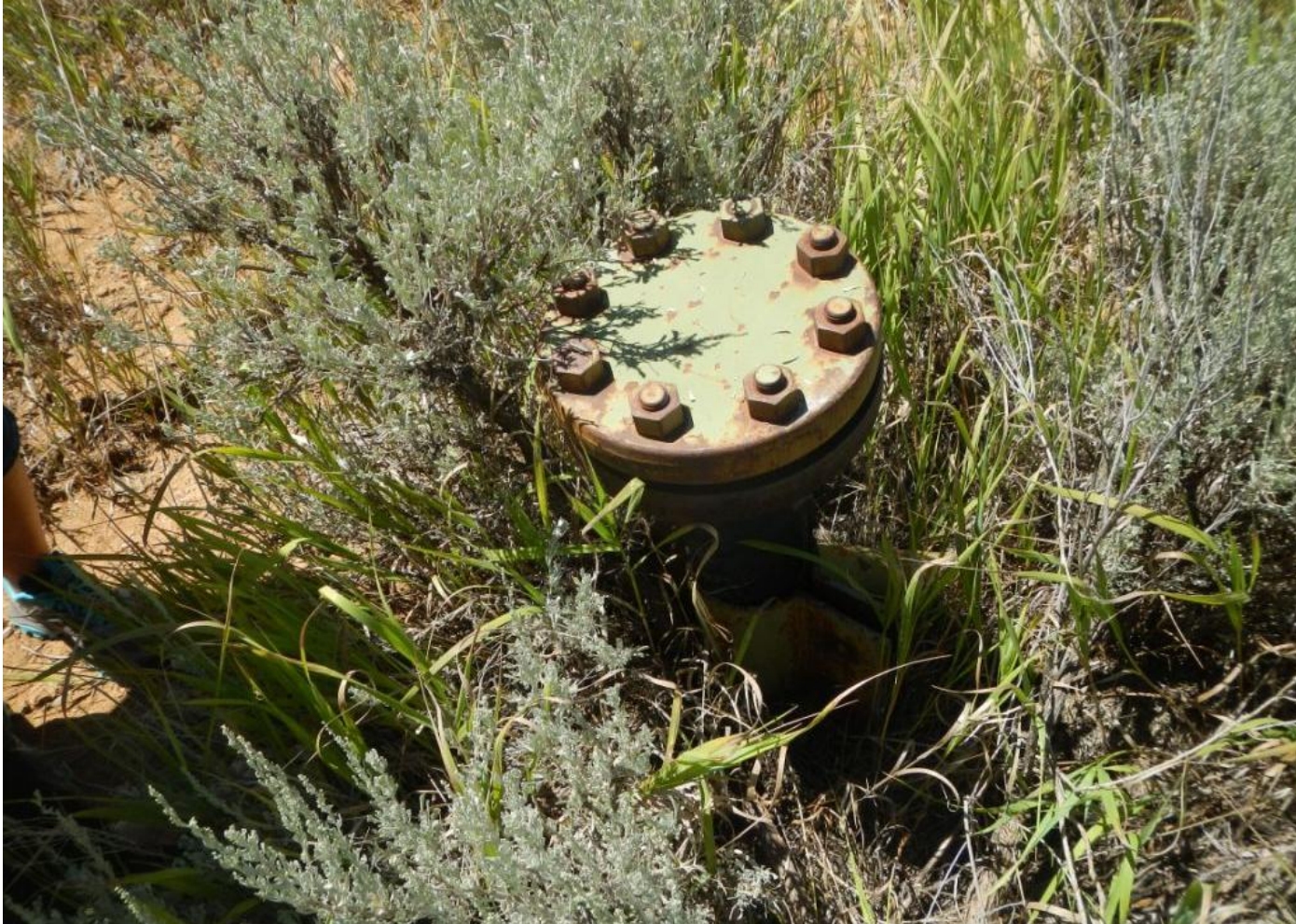
Photo 1. View of riser still in place near the entrance to the well pad.
