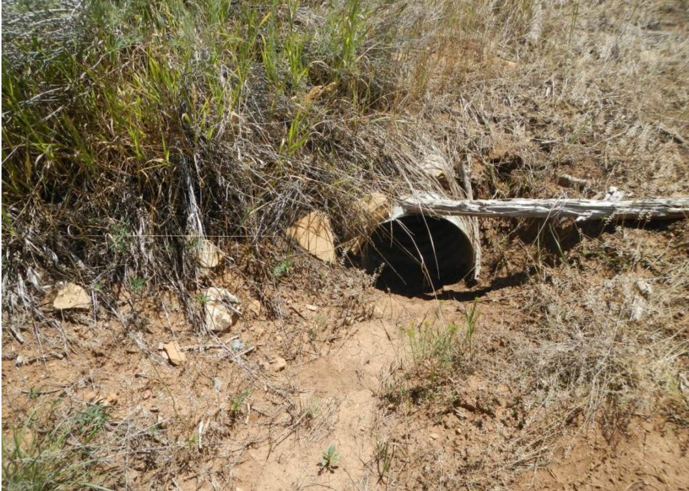
Photo 2. View of culvert in place at the entrance to the well pad.
