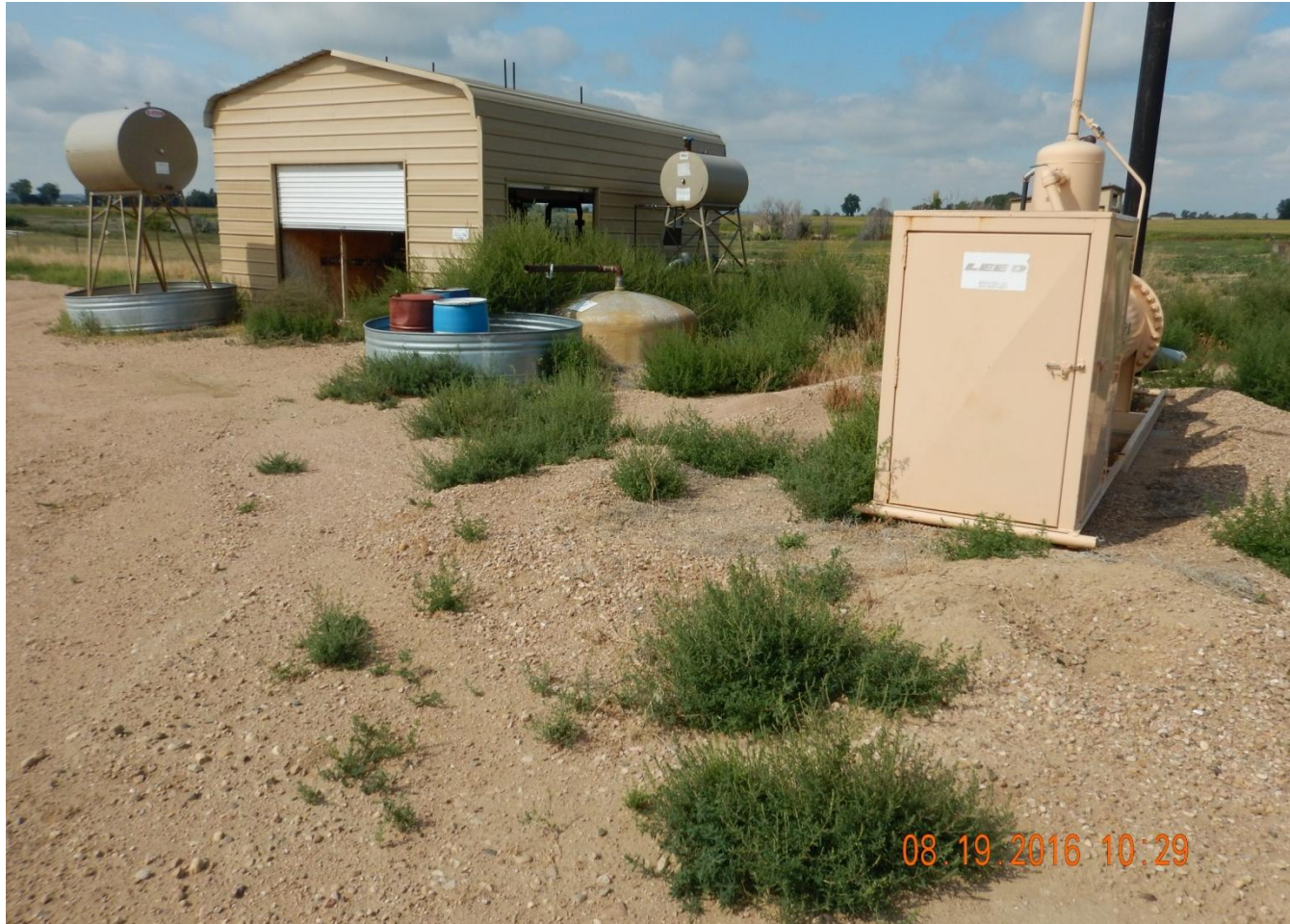
Photo 2. Photo taken from central location, facing Southwest. Control weeds around all equipment at location. Weeds within 25 feet of operating oil and gas equipment are a potential safety or fire concern per Rule 603.f.
