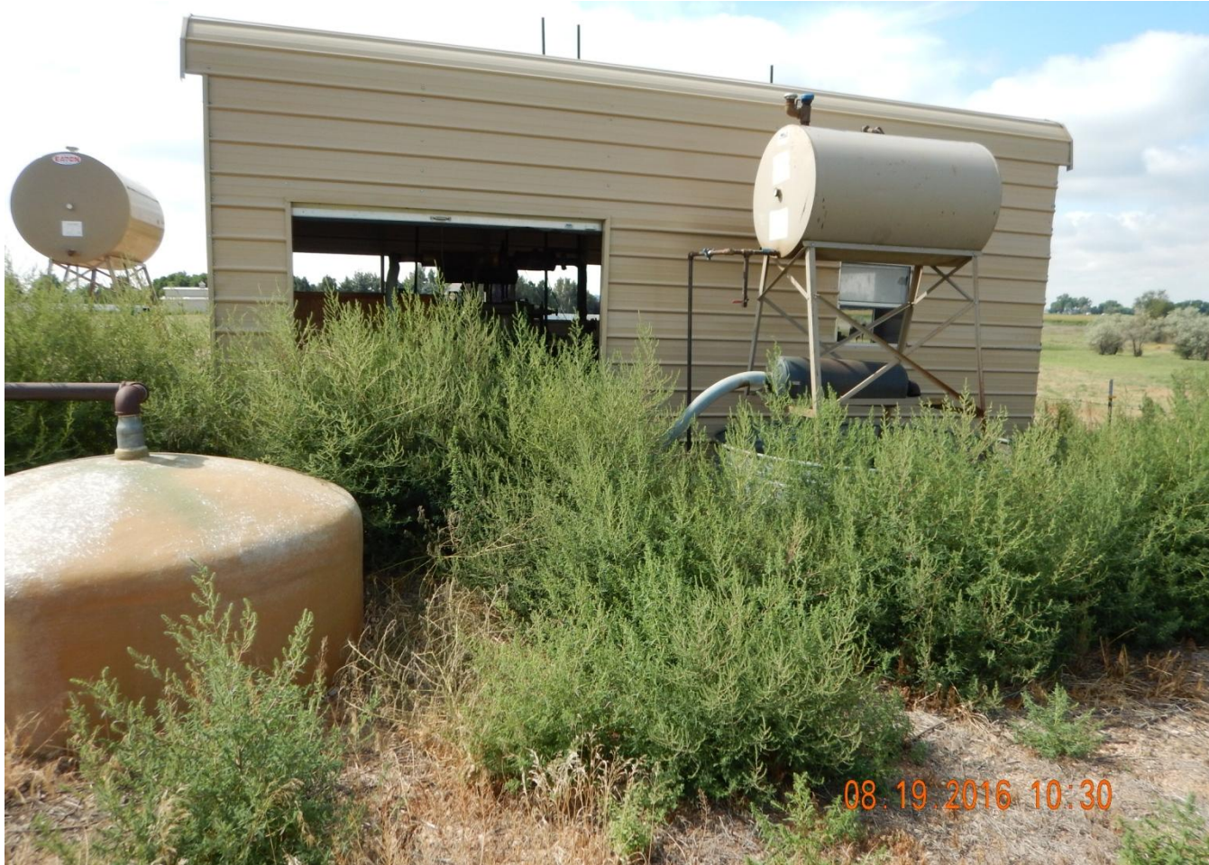
Photo 3. Photo taken from northwestern location, facing South. Control weeds around all equipment at location. Weeds within 25 feet of operating oil and gas equipment are a potential safety or fire concern per Rule 603.f.
