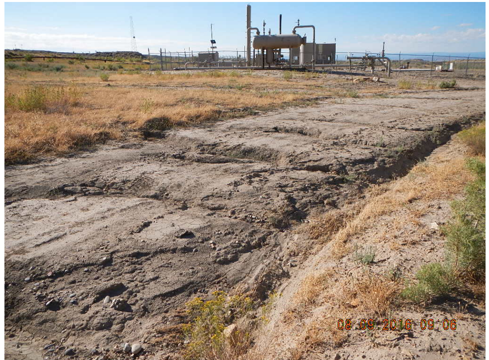
Erosion across access road
