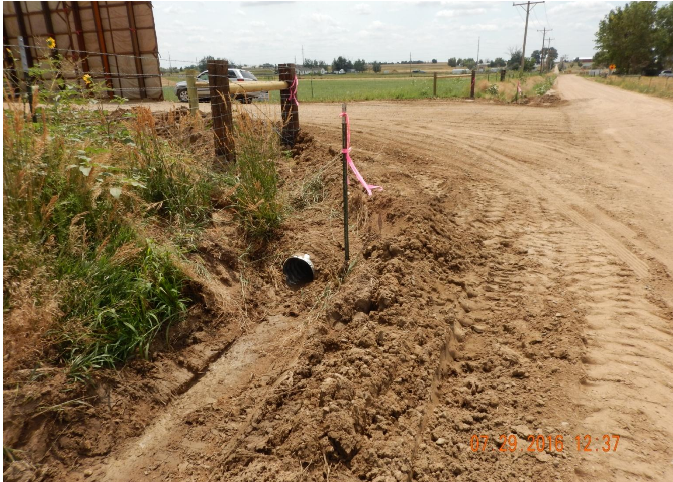
Photo 6. Photo taken from location entrance, facing South. Culvert installed but need to address stormwater and sediment run-on and run-off. Refer to photos 7-8.
