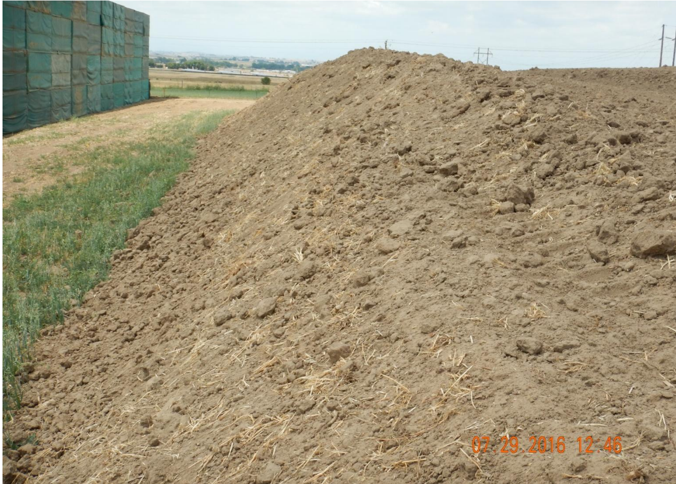
Photo 4. Photo taken from northern location, facing West, towards the south-facing topsoil stockpile. Topsoil stockpile, north-facing and south-facing, sides are steep and could pose erosion issues in the future. In the future, spread out the topsoil stockpile to eliminate the chance of erosion.
