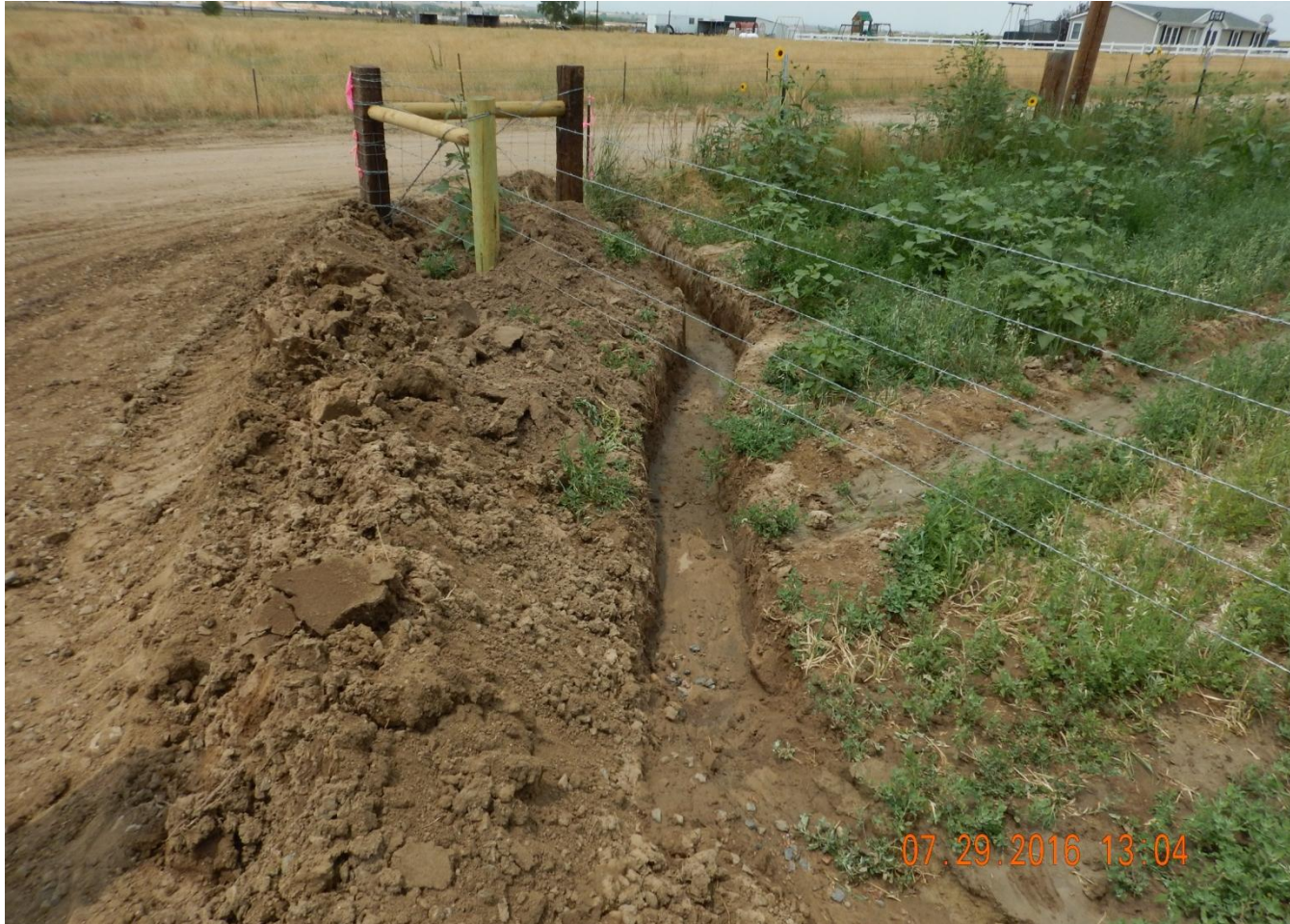
Photo 8. Photo taken from entrance of location, facing West. Temporary ditch was cut but need to install permanent BMPs to control sediment from leaving location.
