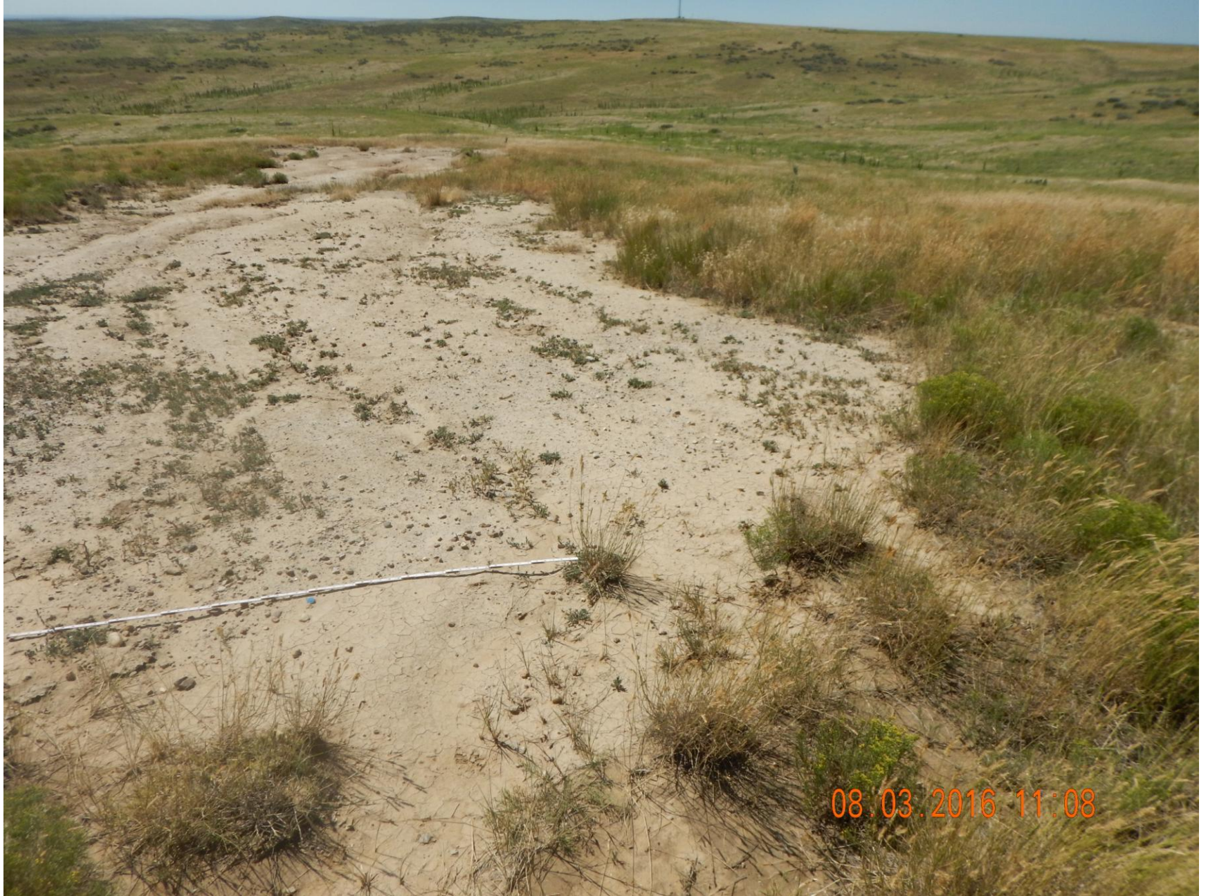
Figure 9: Photo taken from the south end of the location, facing south. Photo shows large un-vegetated area experiencing erosion. Area the result of a produced water spill. 6' measuring stick for reference.
