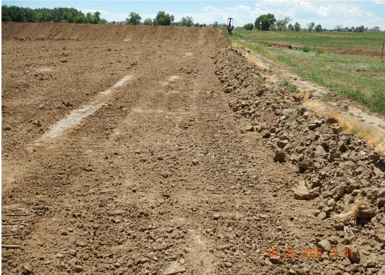
Photo 1. Photo taken from western location, facing South towards topsoil stockpile. Need to stabilize topsoil stockpile upon completion of salvage operations. Unconsolidated berms along perimeter of location need to be compacted.
