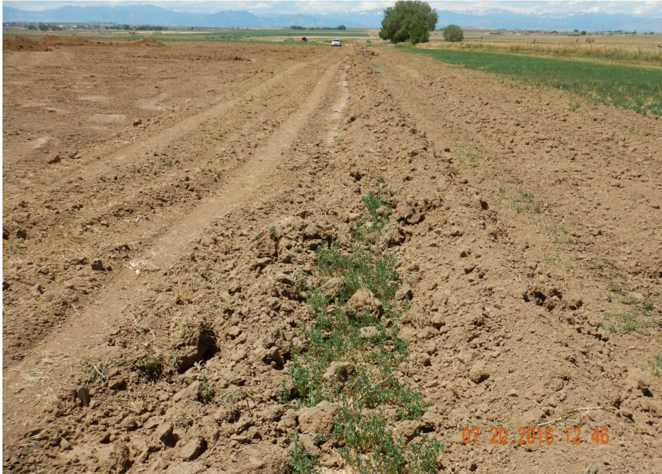
Photo 4. Photo taken from northeast location, facing West. Unconsolidated berms along perimeter of location need to be compacted.
