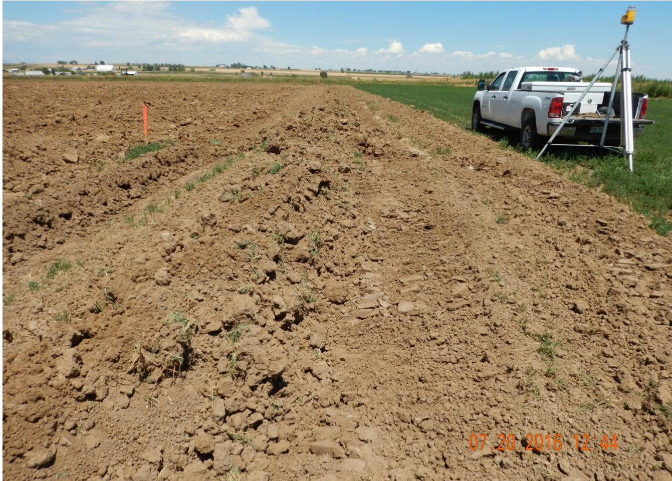
Photo 3. Photo taken from southeast location, facing North. Unconsolidated berms along perimeter of location need to be compacted.
