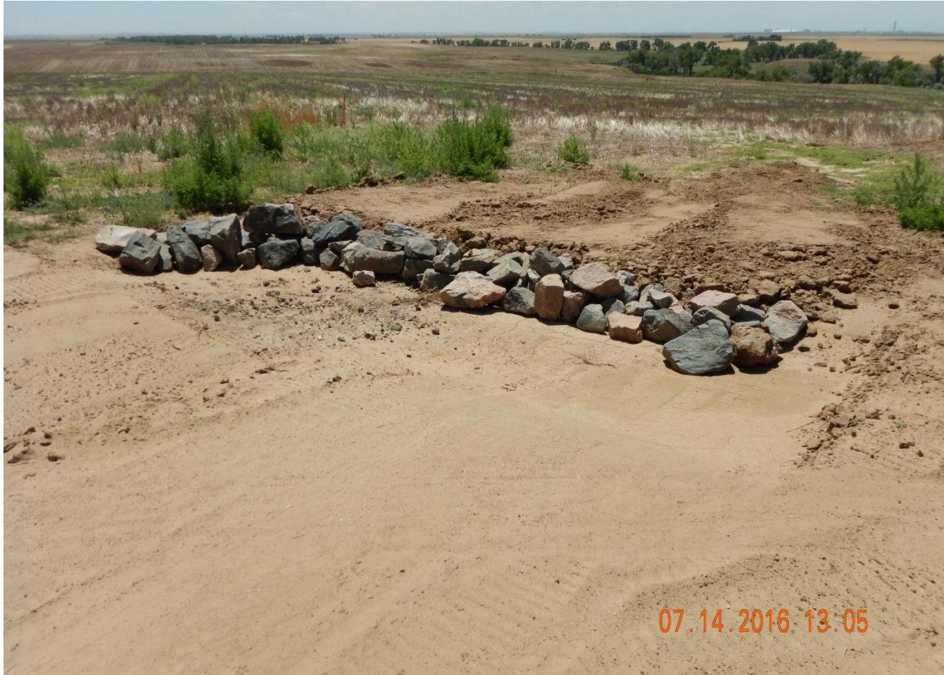
Photo 4. Photo taken from the southern well location, facing West, toward the second BMP. Two stormwater BMPs installed along the southern location to control stormwater and transport of sediment.
