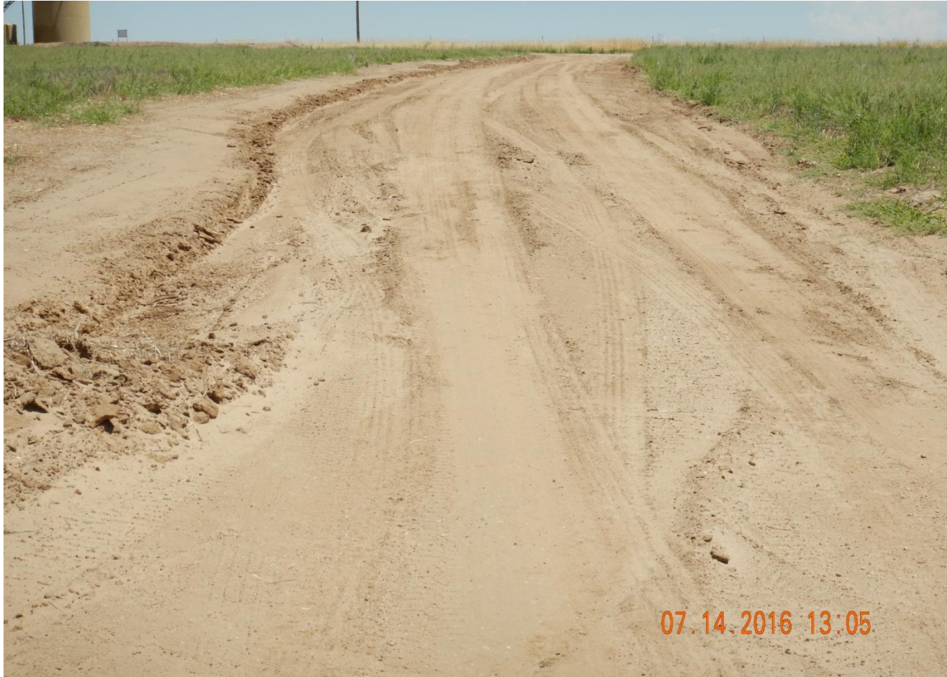
Photo 2. Photo taken from well location, facing East, along the access road. Rills from erosion along the access road have been fixed.
