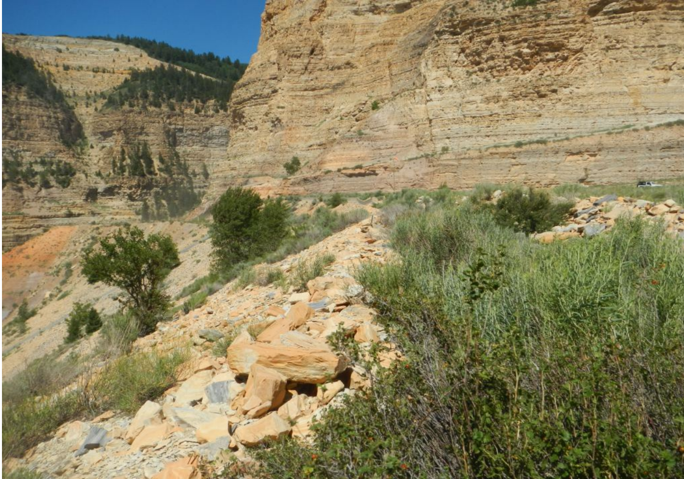
Photo#11: View to West along Fill Slope ditch and Berm at South edge of Location
