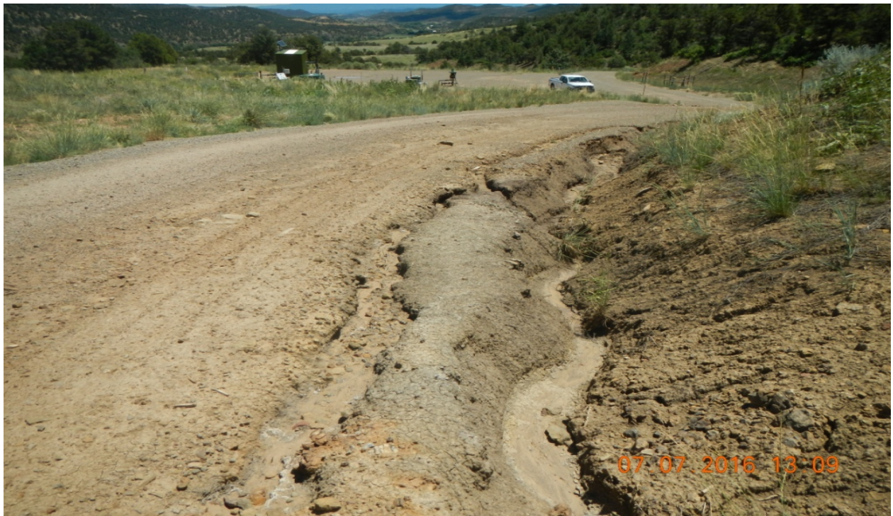
photo 8: There is erosion occurring along the access road west of the location.
