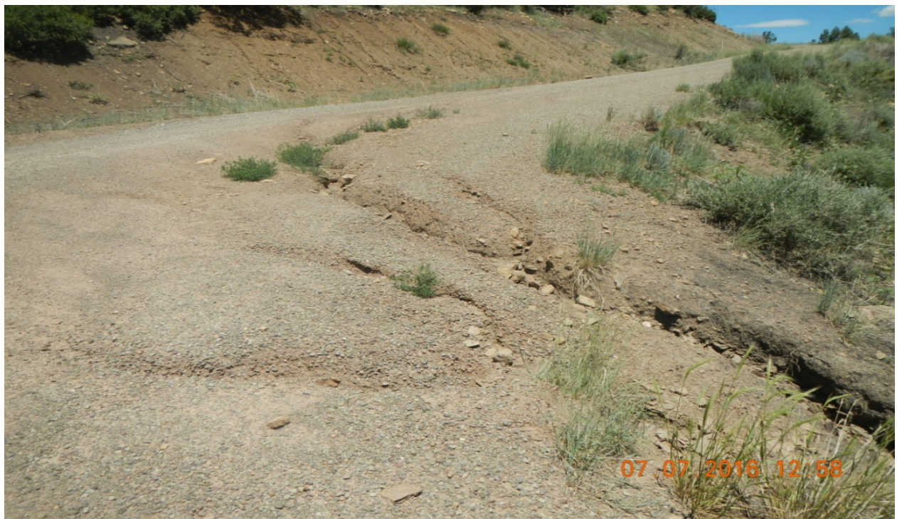
photo 2: Area of erosion along the access road south of the location.
