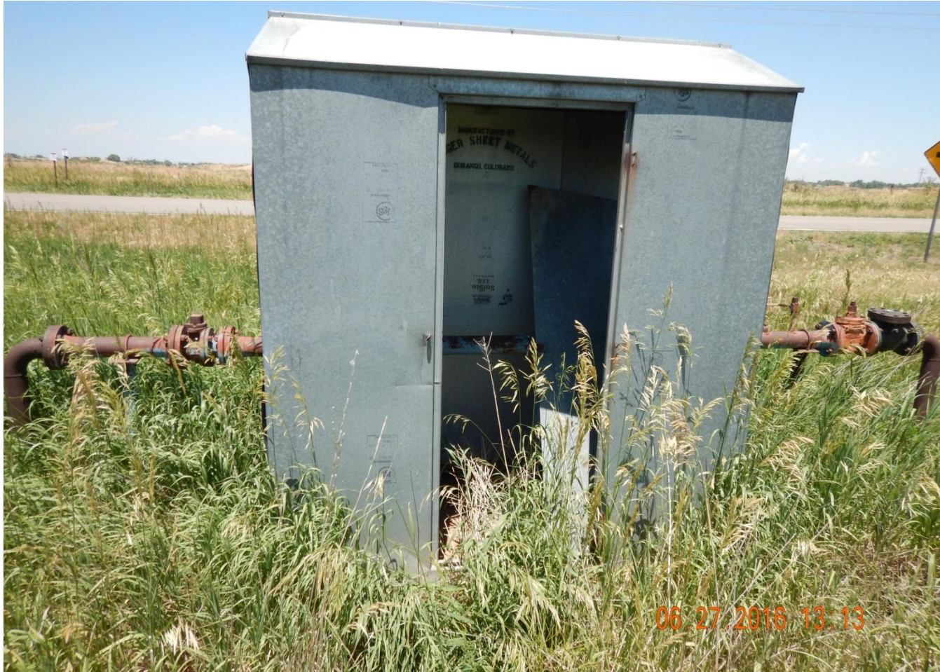
Photo 4. Photo taken from the eastern tank battery location. Equipment still remains and needs to be removed per Rule 1004.
