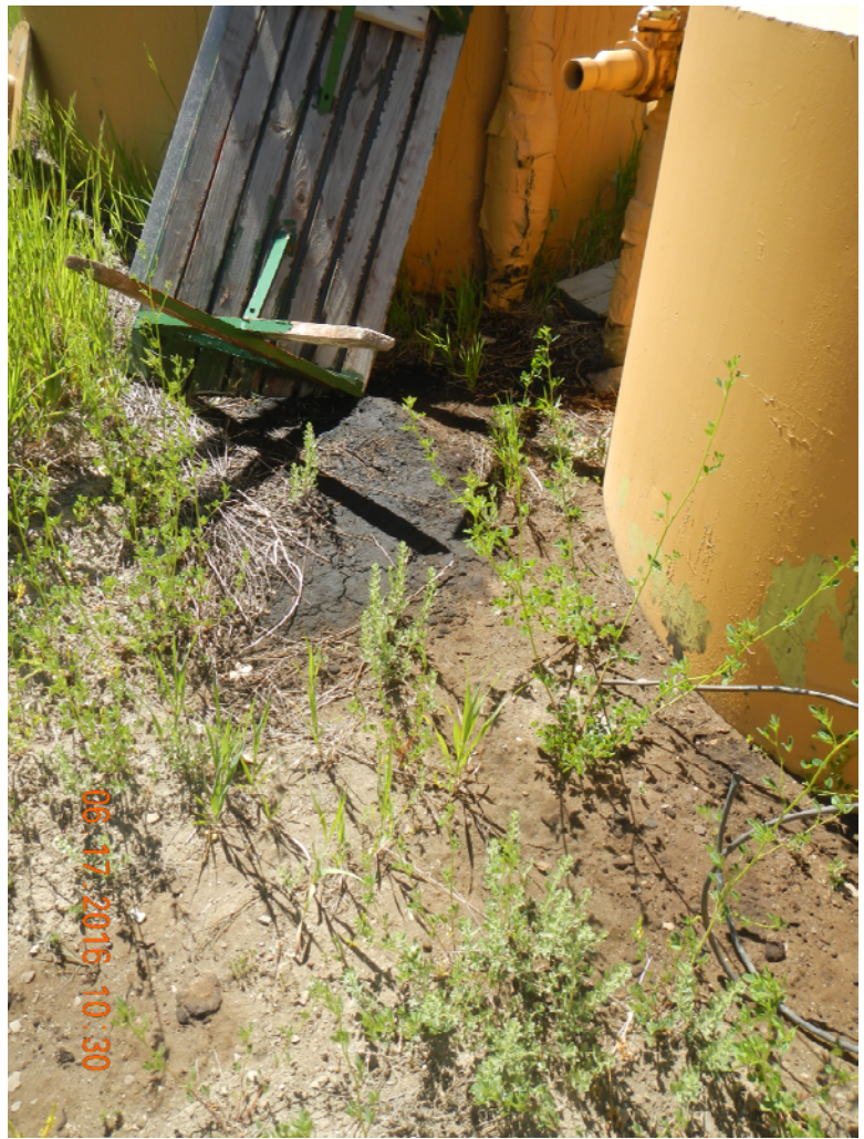
Stained soil from leak at tank base.
