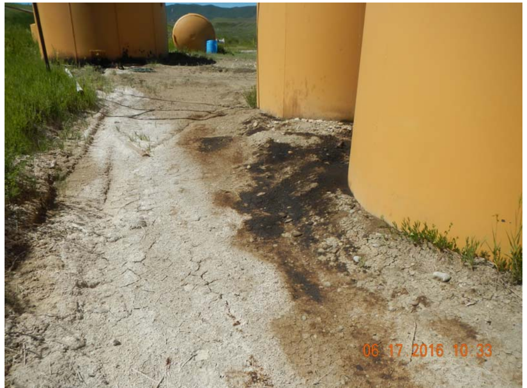
Stained soil at tank bases.
