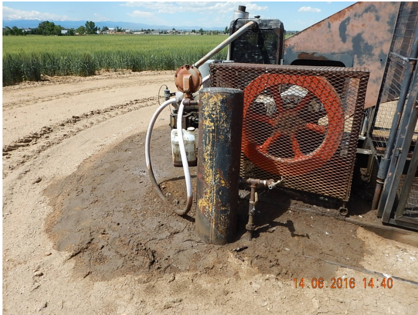
Lube Oil Release Observed at Prime Mover
