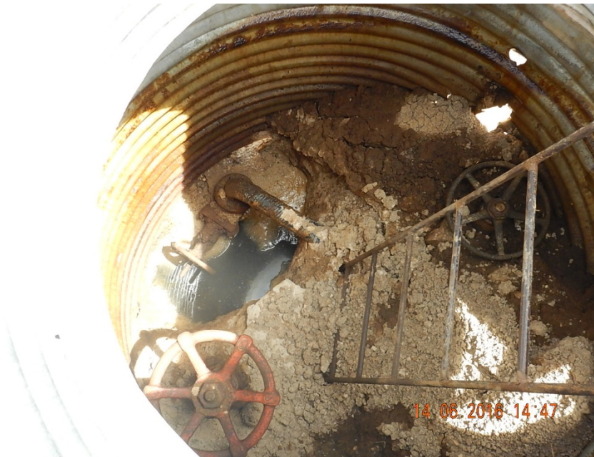
Free crude oil at bottom of valve can
