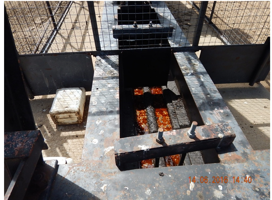
Lube Oil Accumulations Observed Inside Frame Rails of Pump Jack
