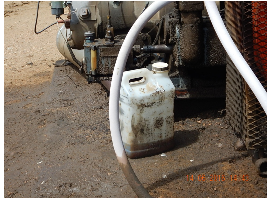
Unlabeled Container at Prime Mover
