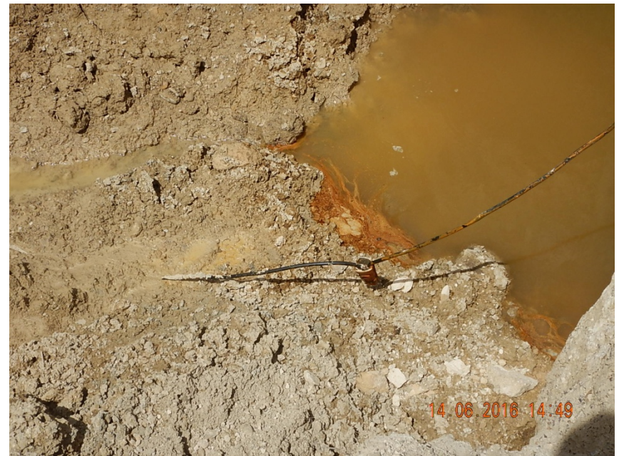
Crude oil residue in stormwater at bottom excavation
