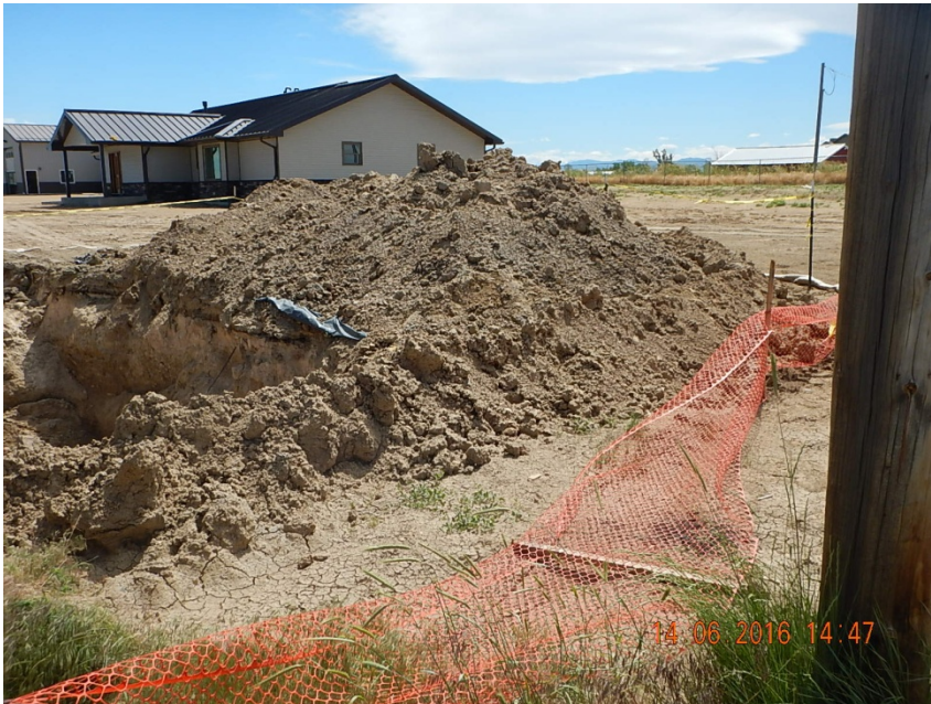
E & P Waste Soils adjacent to excavation/ unmaintained fencing
