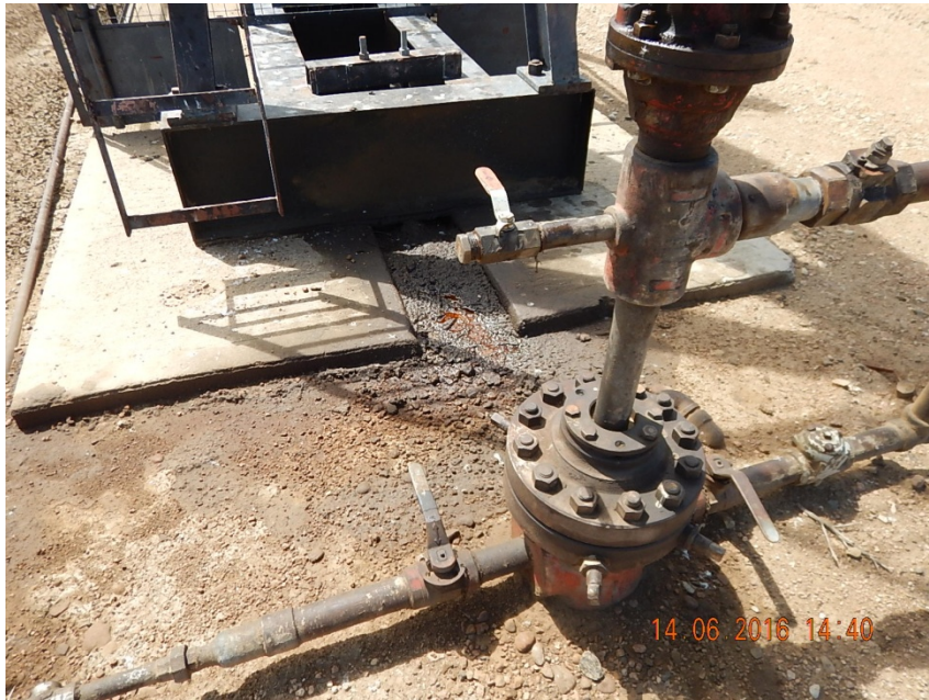
Lube Oil Spill/ Release Observed at Wellhead
