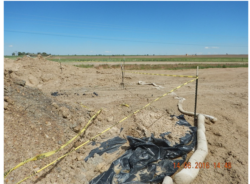
Unmaintained BMP's adjacent to E & P Waste soil pile
