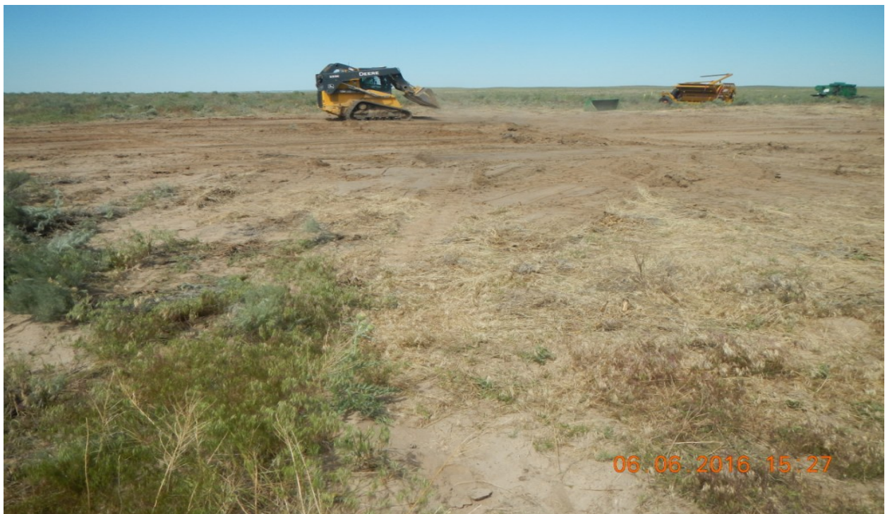
photo 4: Once all the debris was removed the location was releveled and contoured.
