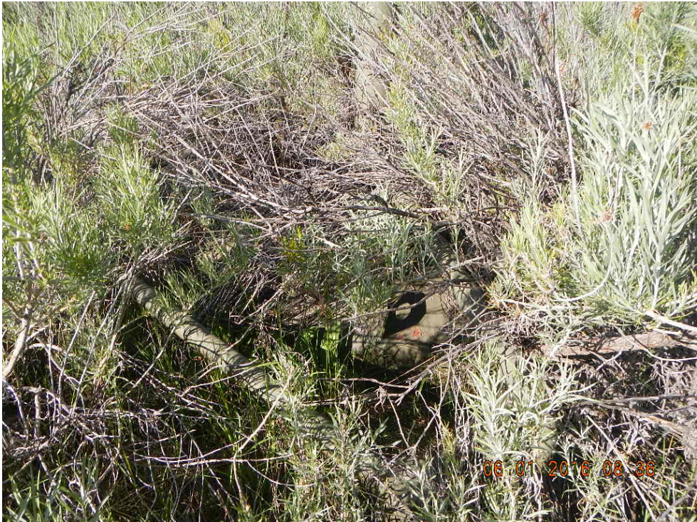
Vegetation around tank and no signage.
