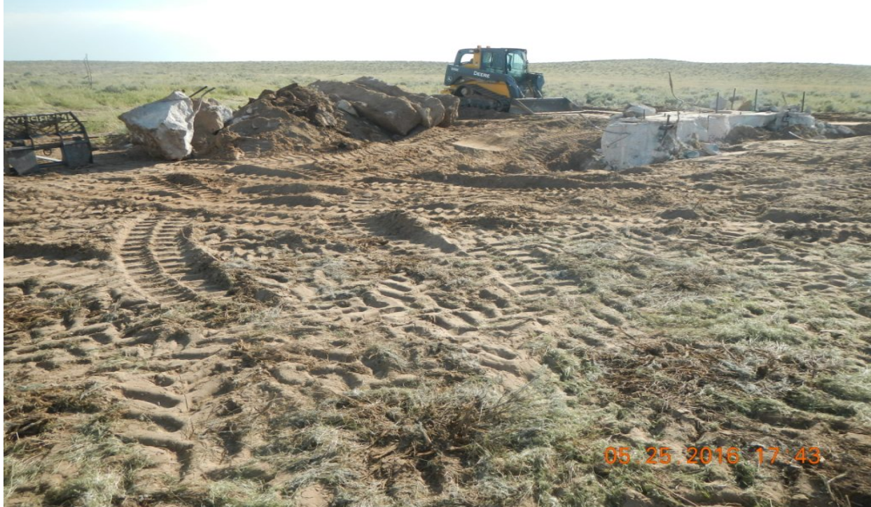
photo 8: Facing southwest toward the cement pad (1) at Lat/Long: 40.08697,-103.68970. Work concluded for the day.
