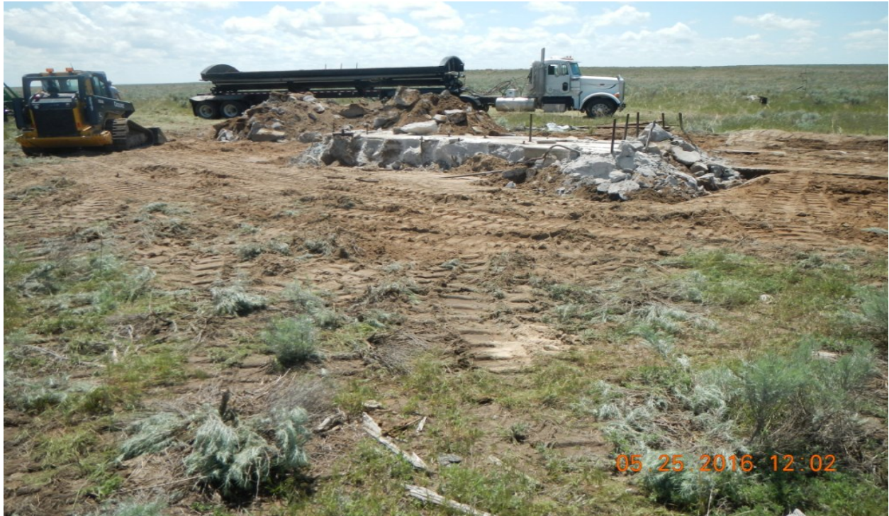
photo 3: Facing south toward the cement pad (1) at Lat/Long: 40.08697,-103.68970. A side dump trailer was brought in to haul the debris away.
