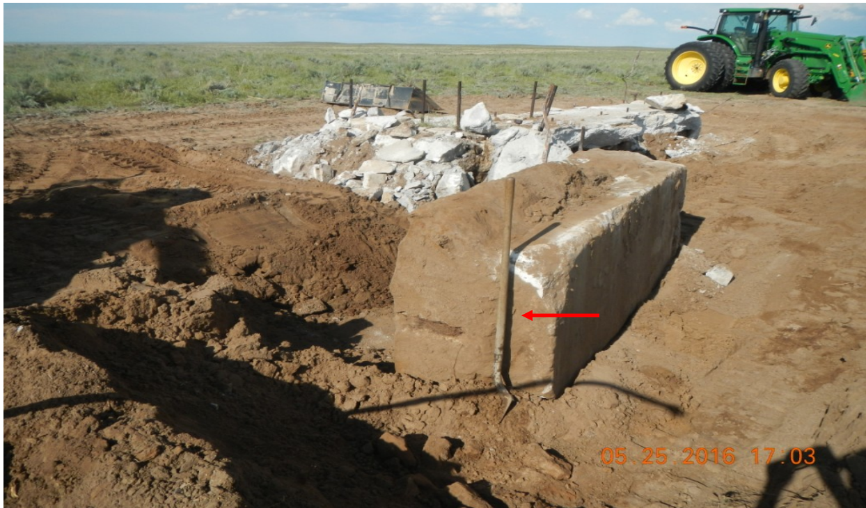
photo 7: The red arrow points to a shovel (4.5 ft.) which shows the thickness of the cement slab (1) at Lat/Long:40.08641,-103.69047.
