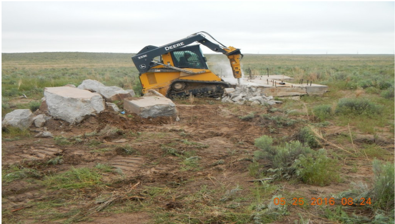
photo 1: Facing west toward the cement pad (1) at Lat/Long: 40.08697,-103.68970. Work began in the morning with breaking apart the cement pad.
