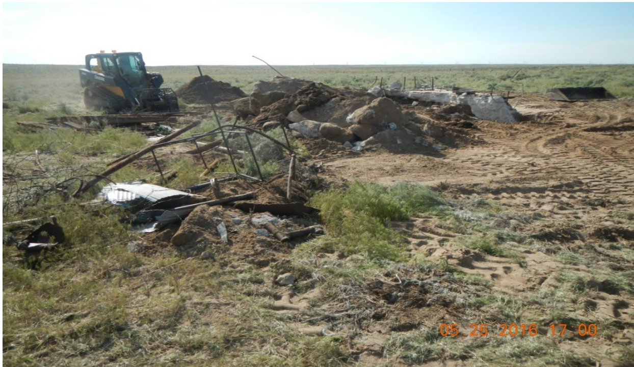
photo 5: Debris piles from cement slab and the various metal and wood debris scattered throughout the location.
