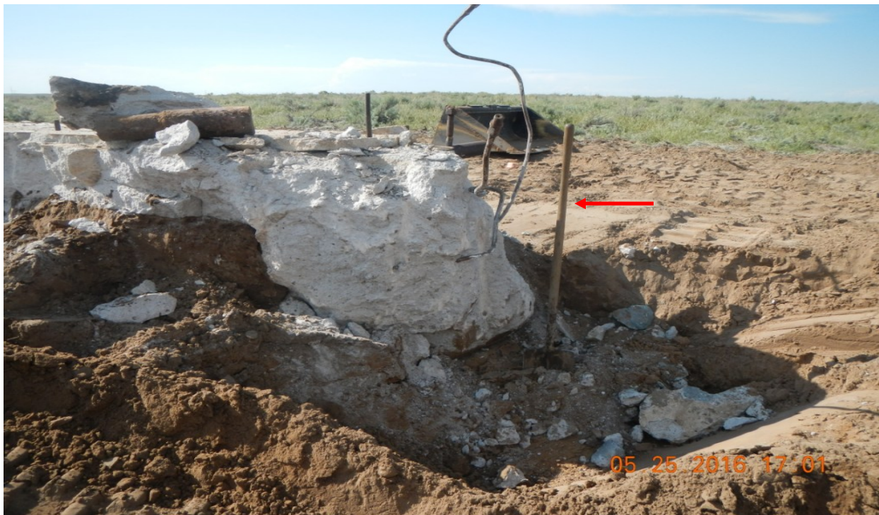
photo 6: The red arrow points to a shovel (4.5 ft.) which shows the thickness of the cement slab (1) at Lat/Long:40.08641,-103.69047.
