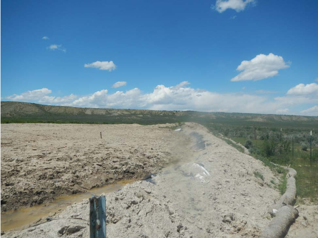
Soil containment area, looking north.
