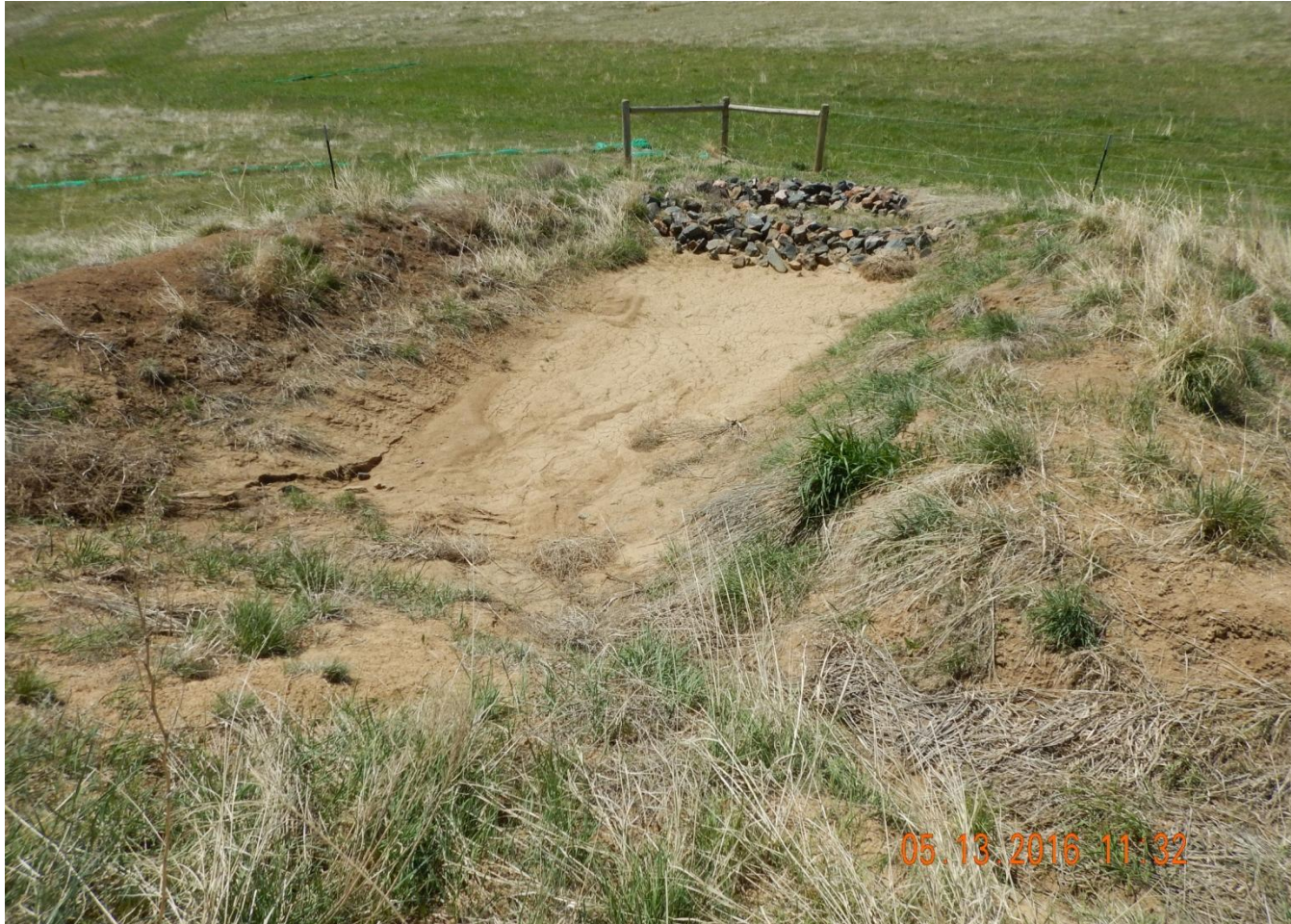
Photo 7. Photo taken from southwest location, facing South towards sediment trap. Sediment trap installed to allow sediment to settle out of stormwater runoff.
