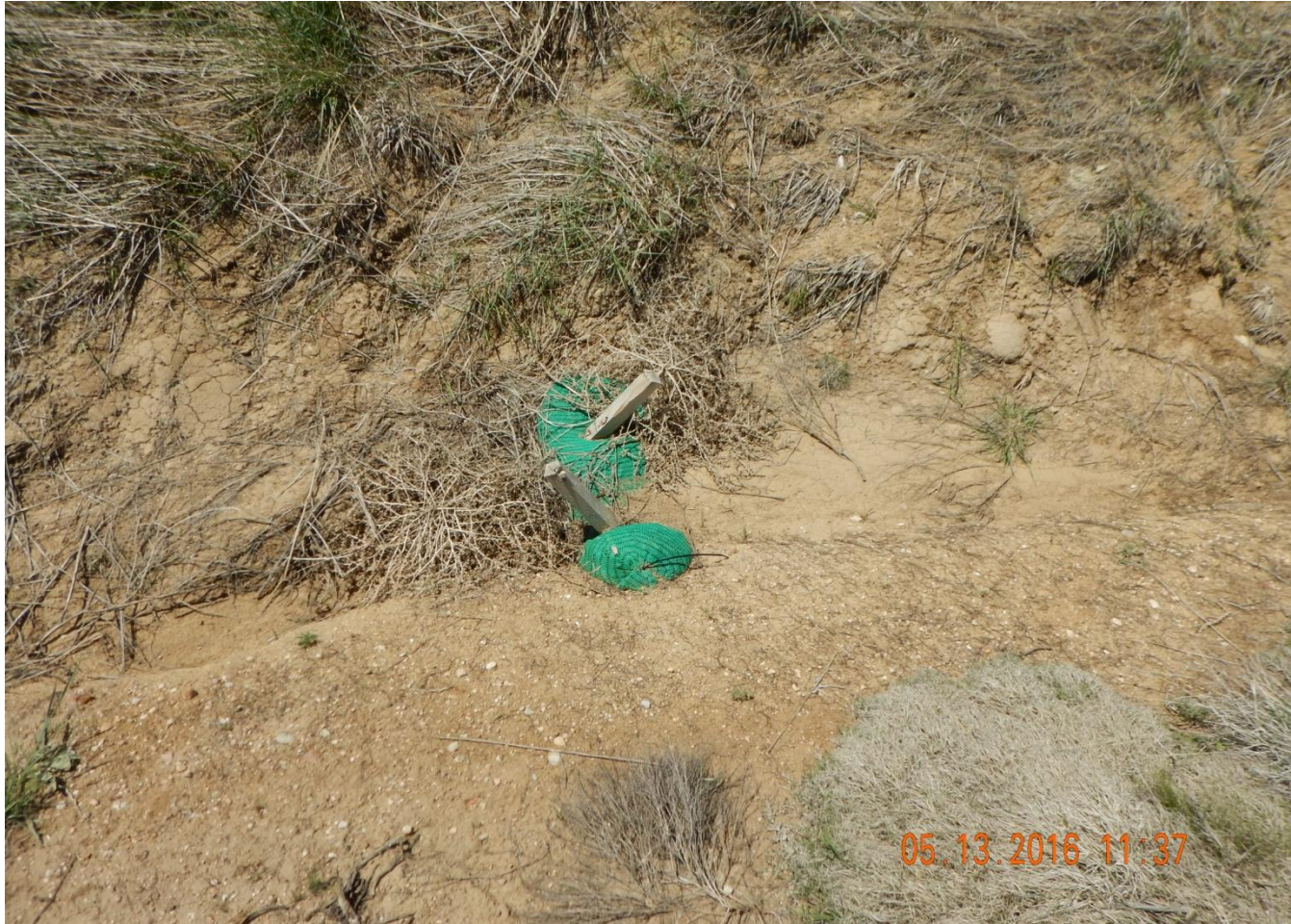
Photo 6. Photo taken from eastern of location. Need to maintain stormwater and sediment control BMPs.
