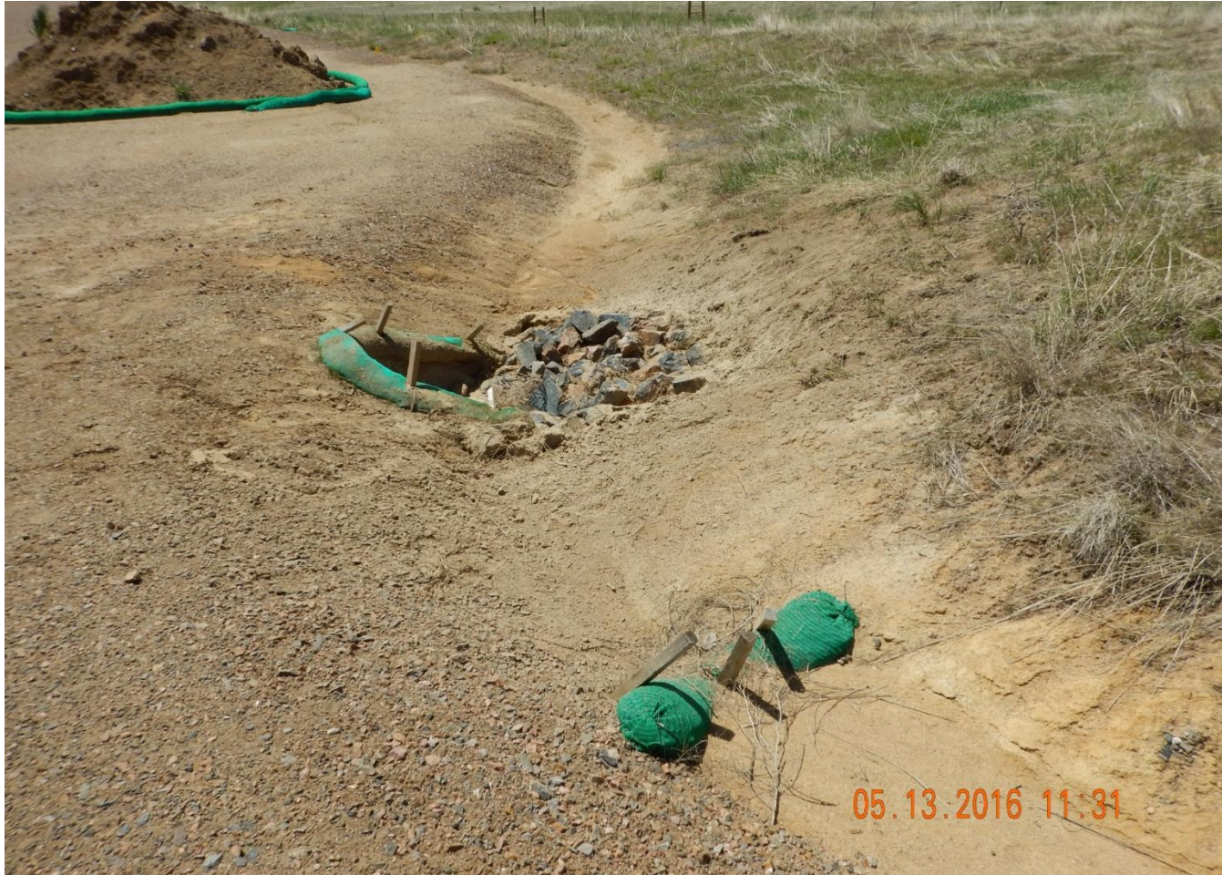
Photo 5. Photo taken from entrance of location, facing South. Need to maintain stormwater and sediment control BMPs.
