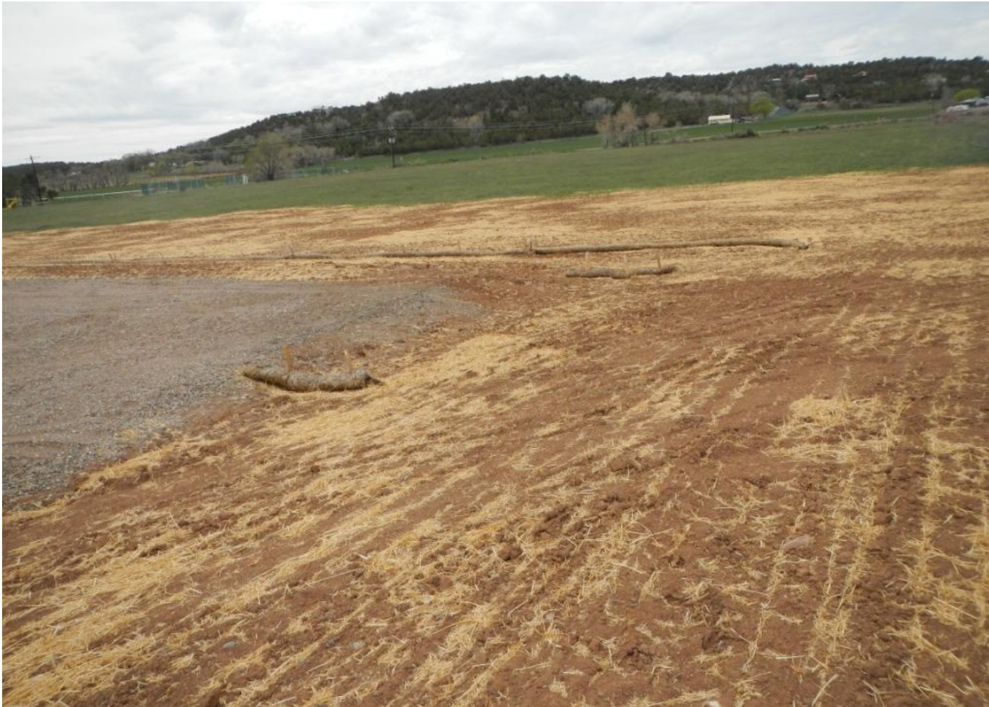
Photo 4. View of wattles and stormwater diversion in the northwestern edge of the working area and the interim reclamation area.
