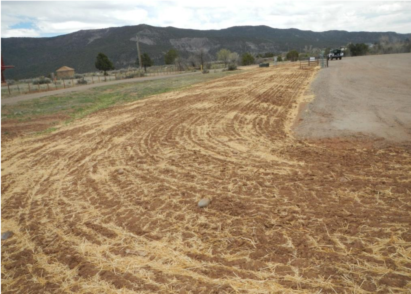
Photo 2. View of the eastern portion of the project area from the northeastern corner facing southward. Interim reclamation has commenced and outer portions of the well pad have been recontoured, decompacted, straw mulch crimped, and likely seeded.
