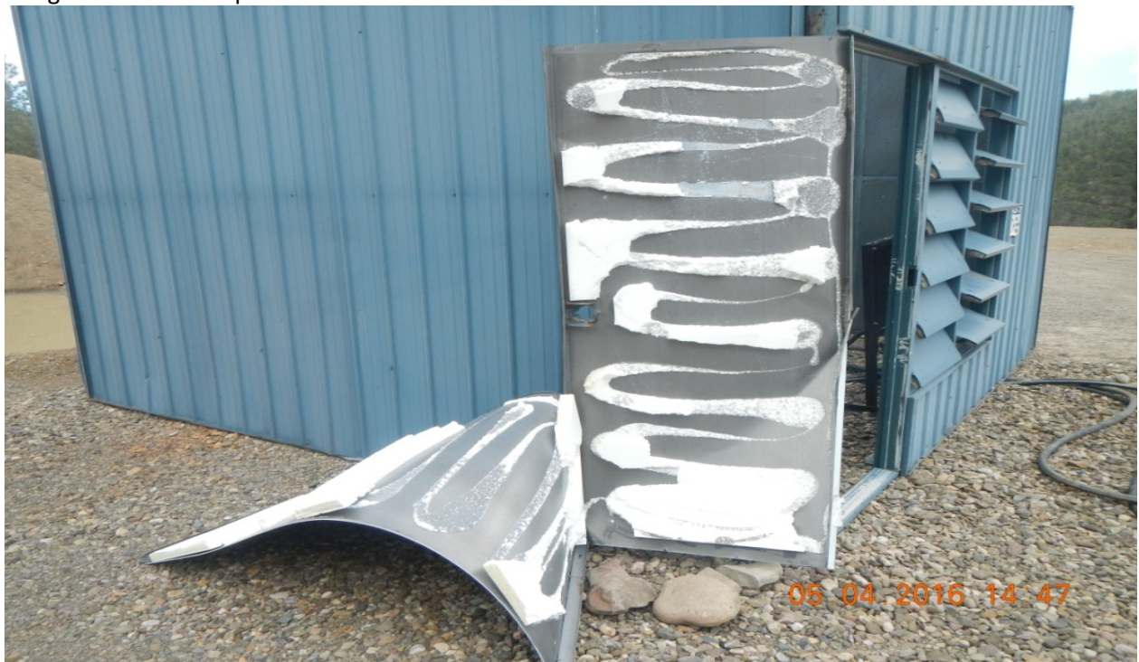
photo 6: Door of the shed is broken.
