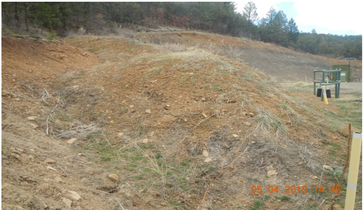
photo 4: Facing northwest toward location. Diversion ditch around the west side of the location.
