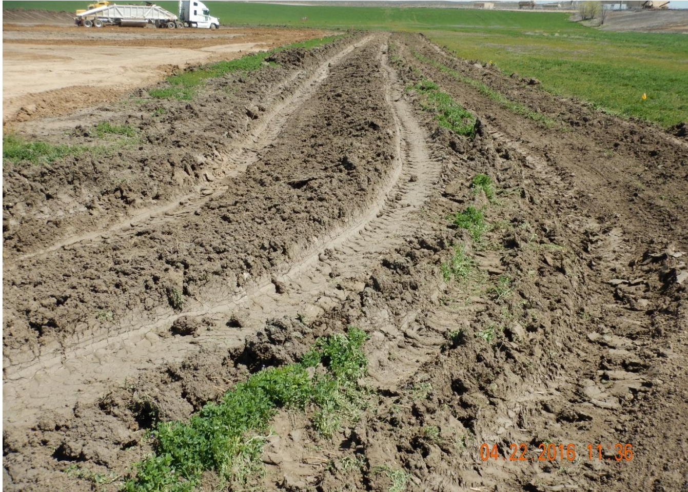
Photo 2. Photo taken from southeast location, facing North. Stormwater control BMP installed in center of photo.
