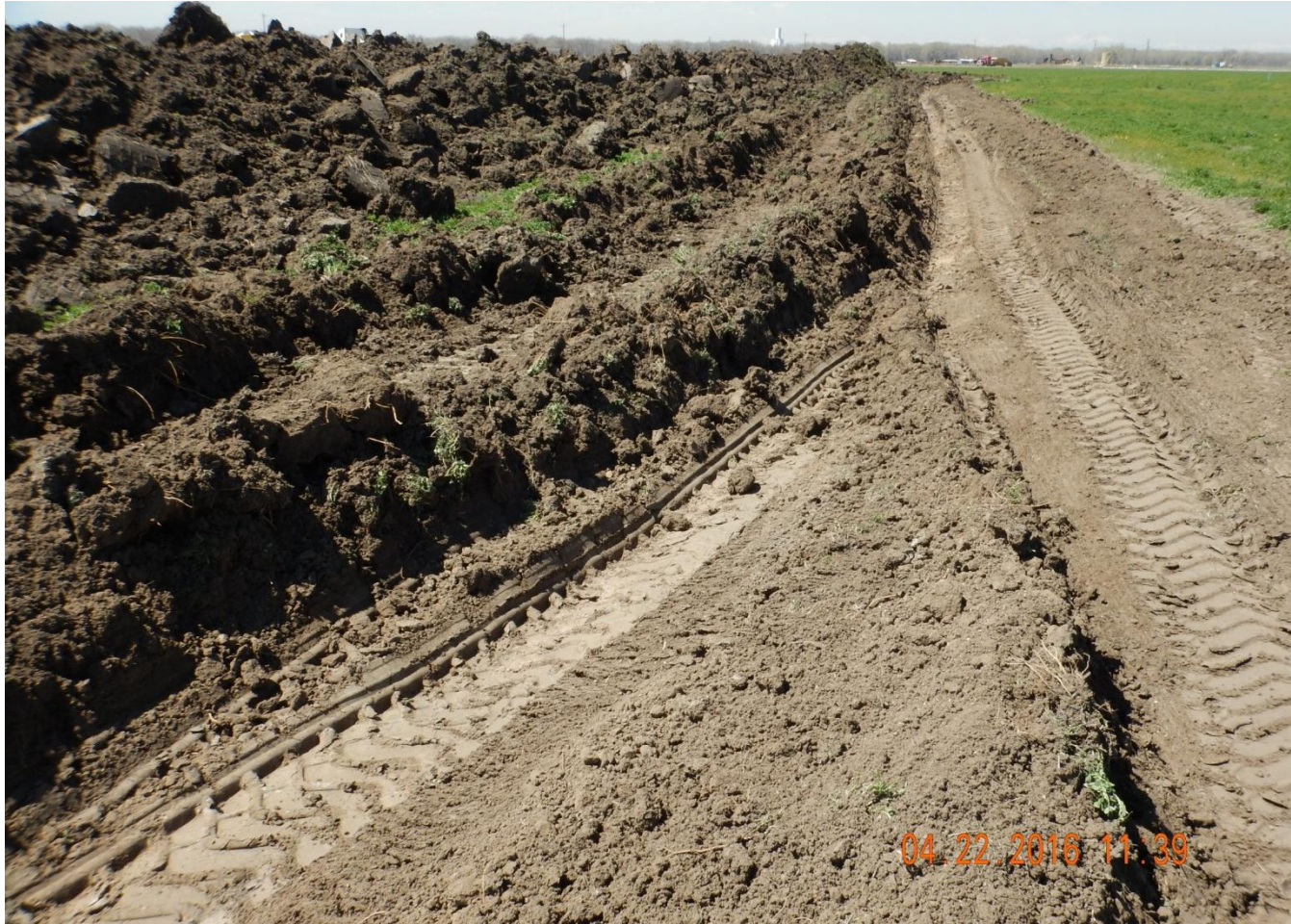
Photo 3. Photo taken from northeast location, facing West. Stormwater control BMP installed in center of photo.
