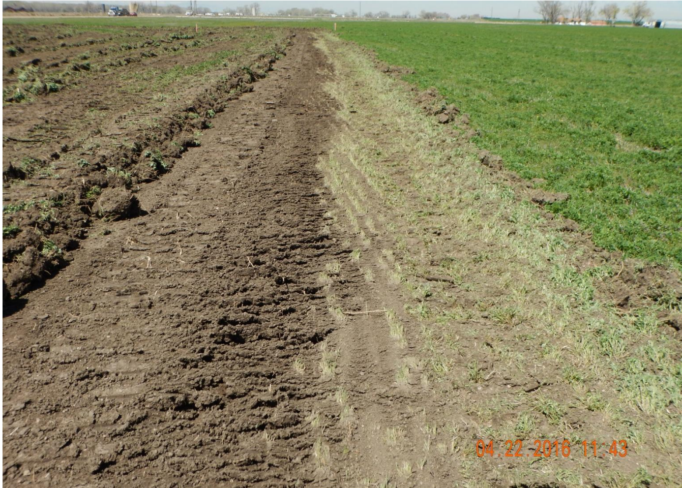
Photo 5. Photo taken from western location, facing West. Stormwater control BMP installed in center of photo.
