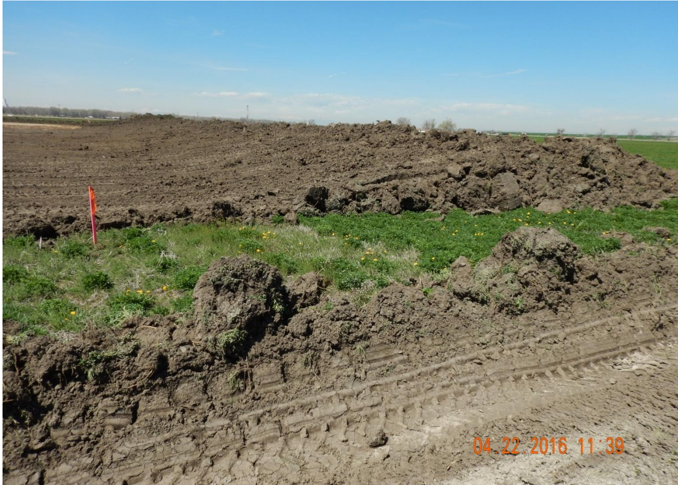
Photo 7. Photo taken from eastern location, facing West towards topsoil stockpile. Topsoil stockpile needs to be stabilized upon completion of salvage process.
