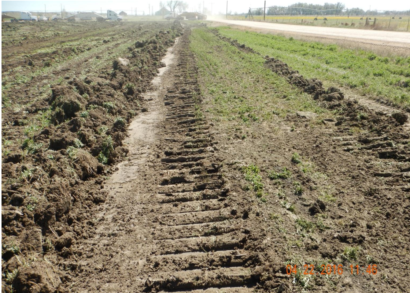
Photo 6. Photo taken from southwest location, facing East. Stormwater control BMP installed in center of photo.
