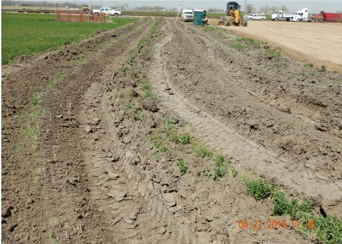
Photo 1. Photo taken from southeast location, facing West. Stormwater control BMP installed in center of photo.
